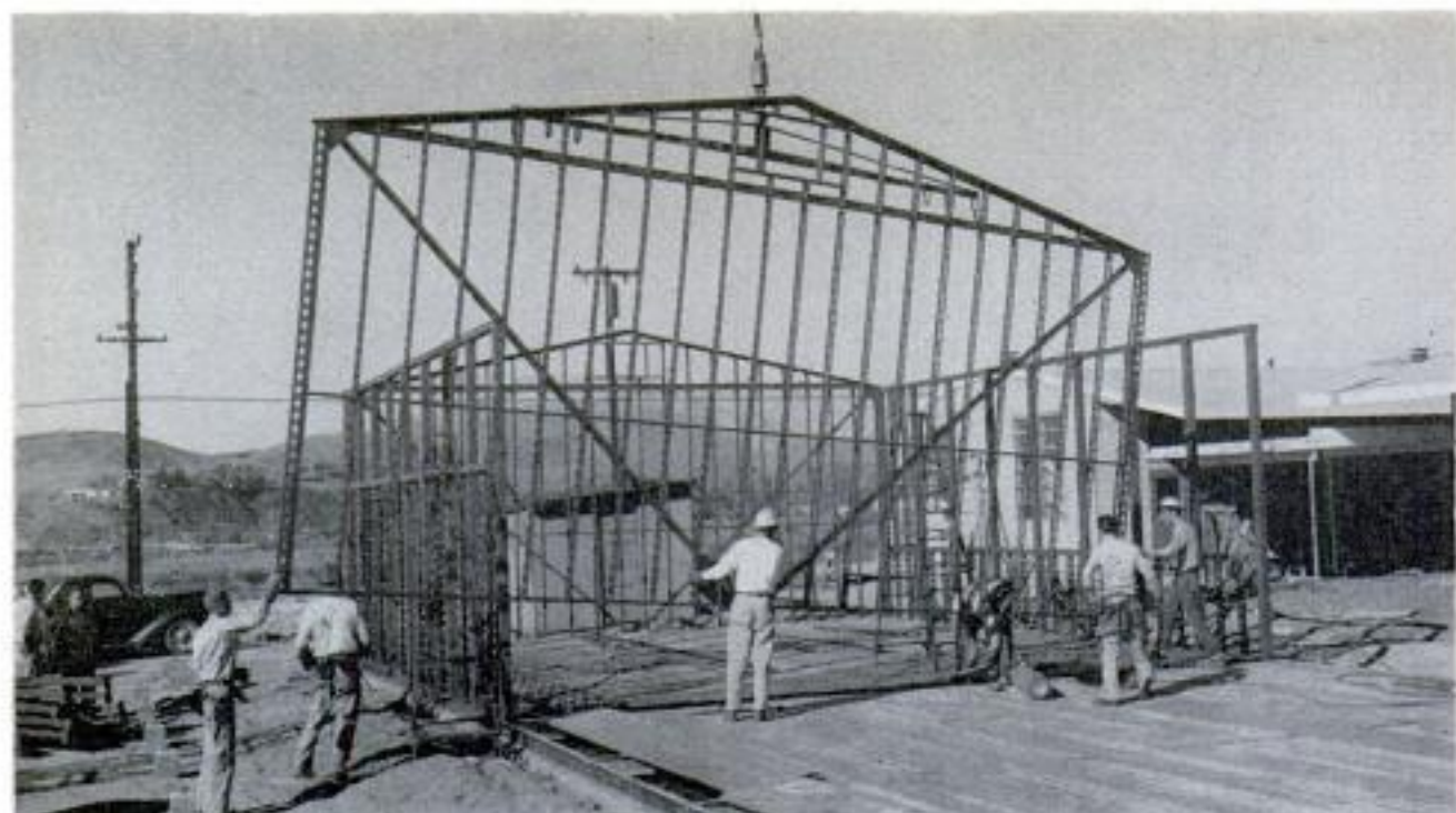
Lightweight steel framework of building goes up quickly. The finished unit can be transported in one piece
