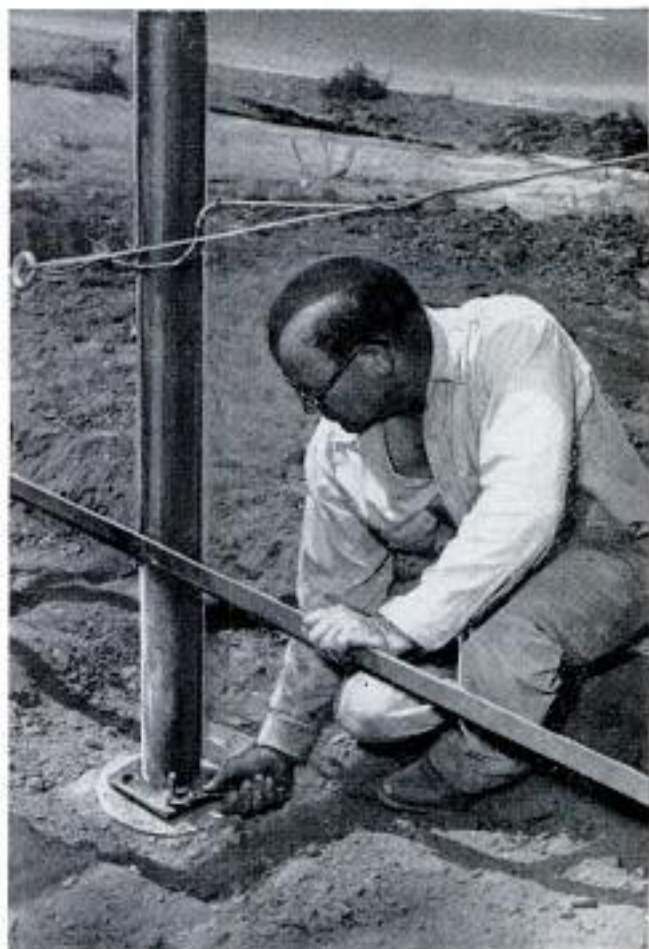
Columns are bolted to concrete piers. Later, footings will be poured around columns up to metal bar
