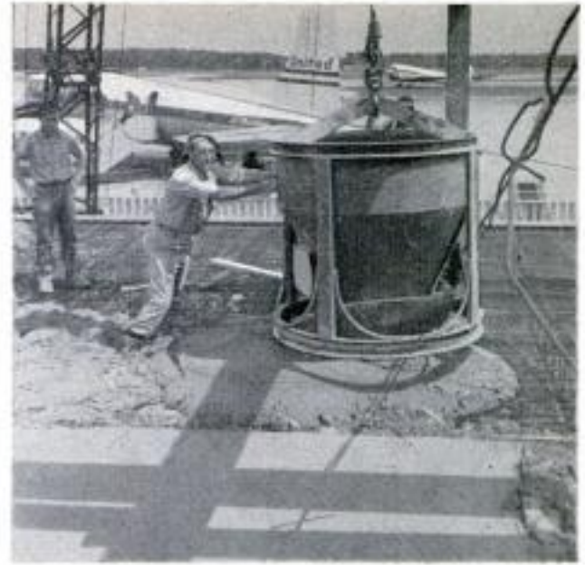
Perlite concrete poured over metal lath becomes lightweight roof deck and insulation for hangar
