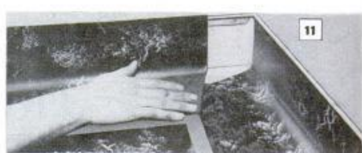
Figs. 11 and 12 show how an inside corner is cut and fitted when metal or plastic corners are not used
