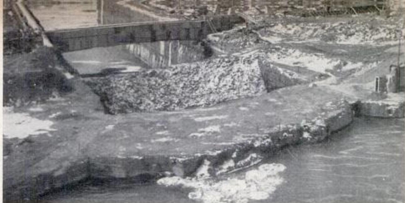
Rock plug separating forebays was loaded with 12,000 pounds of explosives. Power station was 160 ft. distant
