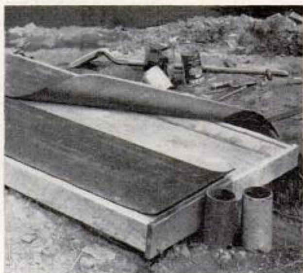
Lid sections are covered with roll-type roofing to seal tank from surface drainage. A narrower strip of roofing is laid over seam formed by first two pieces. Standpipes in foreground lead to valves
