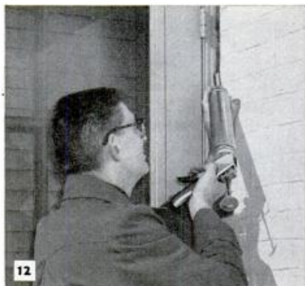
A regular calking gun makes the task of preparing the exterior for repainting easier and quicker
