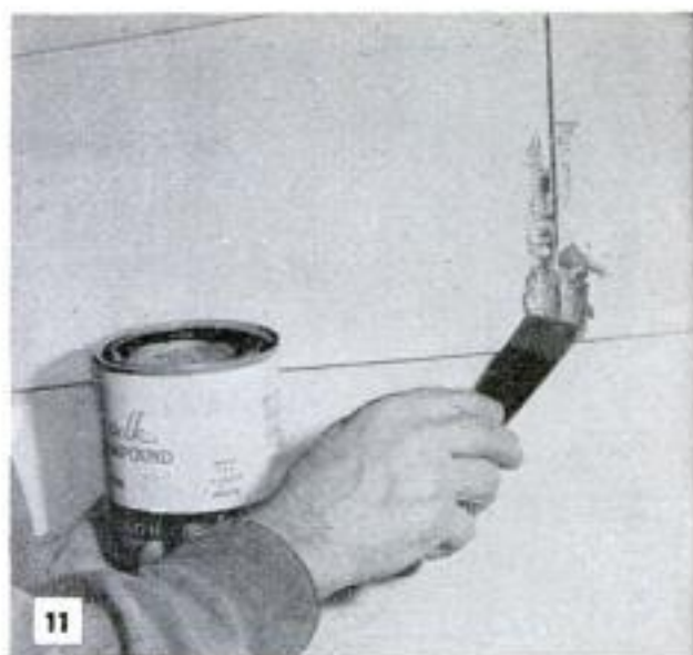
11 Calk all cracks along door and window frames and where wood meets masonry. Get compound in deep
