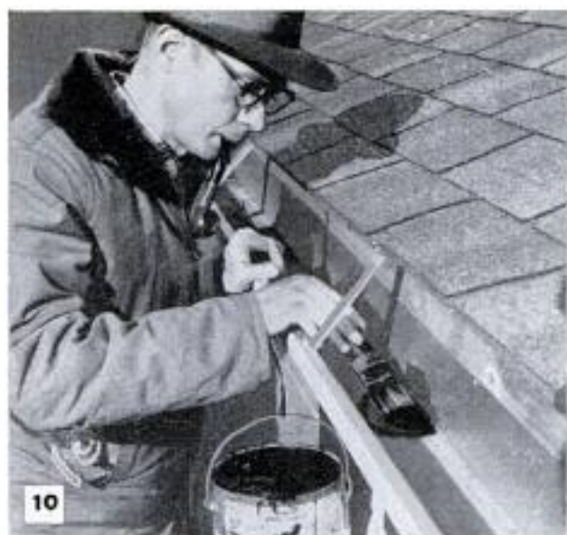
10 Gutters and downspouts should be cleaned and repaired. Paint with roofing cement to preserve, patch
