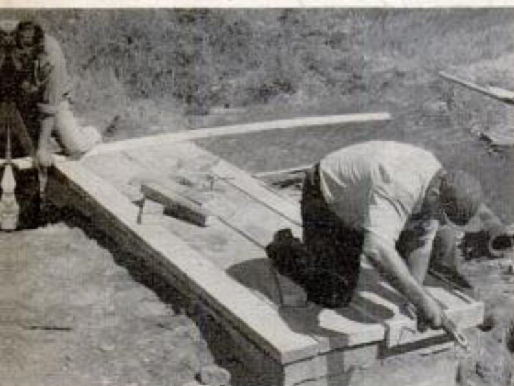
Water supply must be kept clean and protected from contamination, so tank is covered with 2-piece lid of 2-in. planks. Ends and sides of planks are being faced with boards, above, which held lid in position
