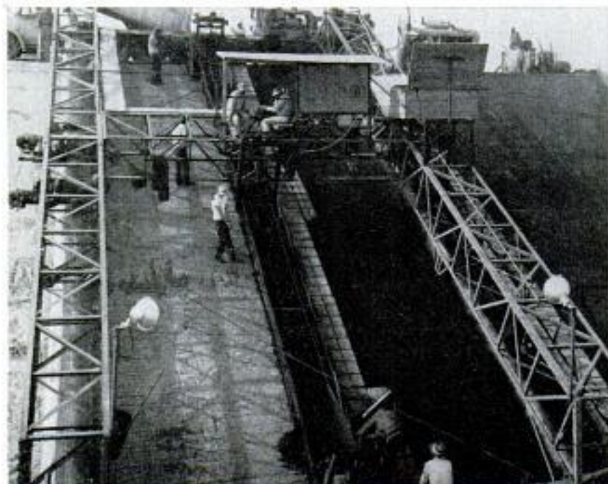
Men with hooks lift wire mesh so that it is embedded in center of asphalt
