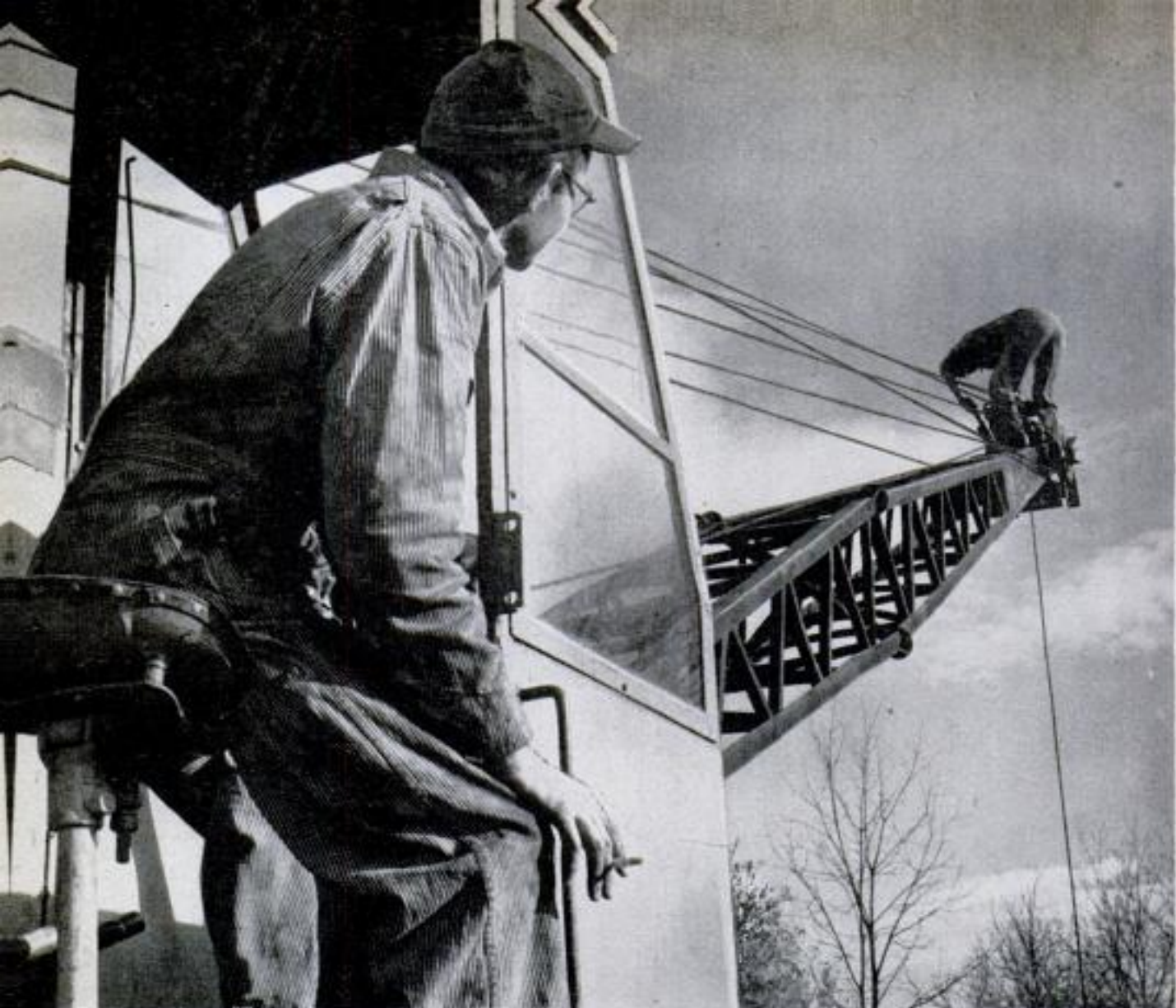
Five dump trucks stood idle until Hamlin climbed out on the end of this crane to unsnarl jammed cables
