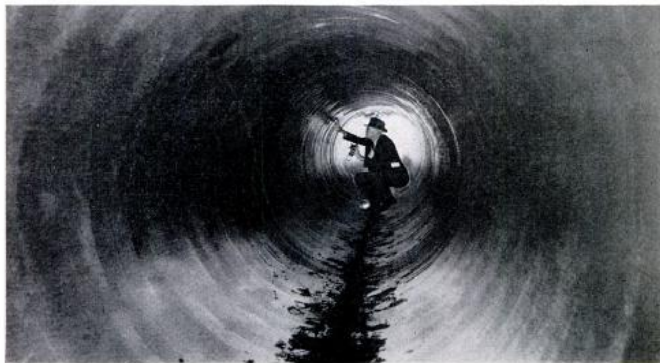
After cleaning with a go devil and lining with mortar, the pipe shown at top of page looks like this
