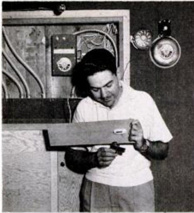
Tamkin tests efficiency of fire-detecting unit at alarm "station" in garage. Each room has one unit
