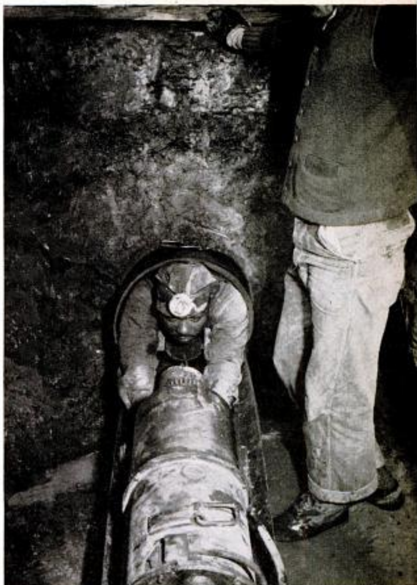
Pipe worker riding contoured "buggy" worms his way into a 16-inch pipe with automatic liner. He will come out feet first
