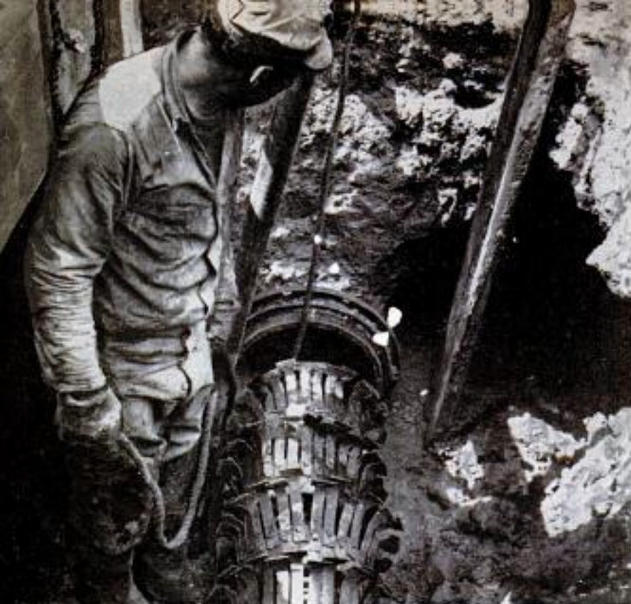
Pipes are cleaned with a "go devil" which has hoelike blades and is flushed through pipe (below) to scrape interior clean
