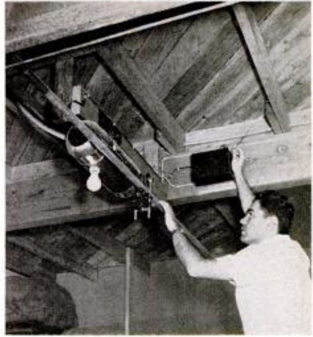
Radio-operated mechanism in garage opens or closes doors when signal is received from approaching car
