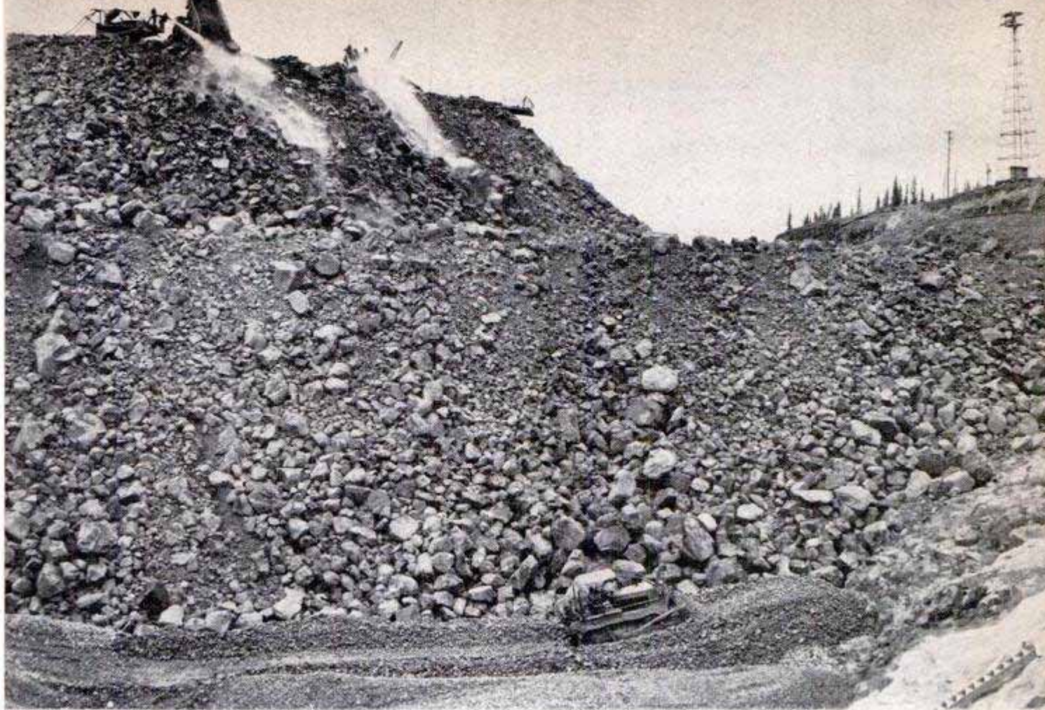
Forty dump trucks shuttled back and forth on 12-minute round trips with rock loads blasted from the slope
