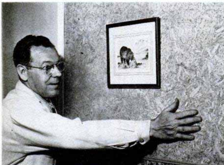
Smooth-finish panel results when surface is impregnated with water putty and sanded down. Tinted putty gives desired color—here, a light pink
