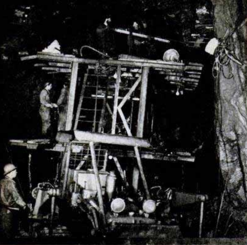
Working in damp tunnels and caverns of jagged rock, drilling crews pushed along at a rate of nearly 300 feet per week in some places. About 260,000 cubic yards of rock were blasted for the underground powerhouse
