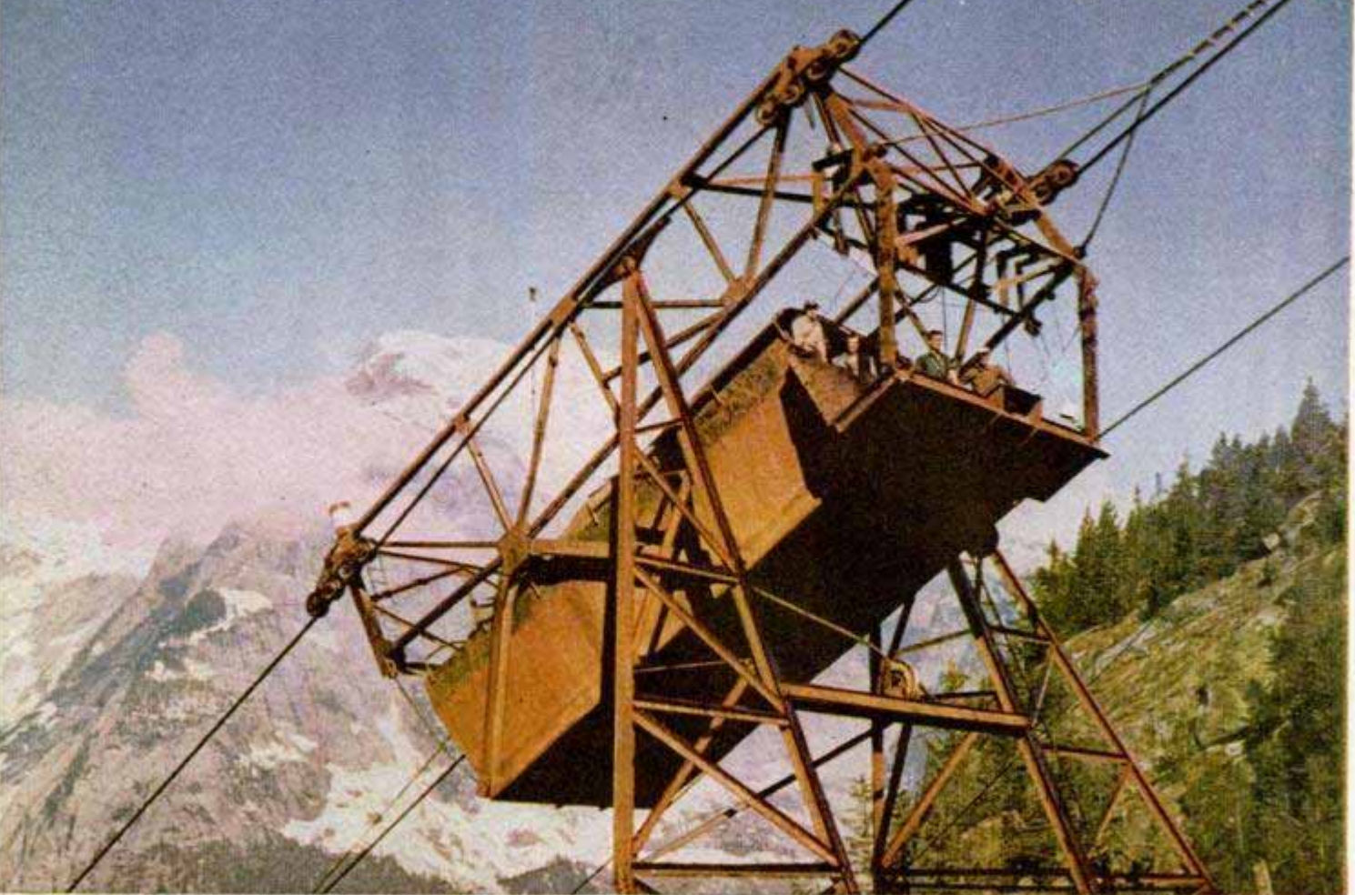
Bulky pieces of construction equipment were moved up the slope, at a 30-degree angle, in this nine-ton cable car
