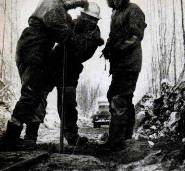
Men carefully tamp a charge of dynamite into a shot hole. Wire will link the detonator to shooting truck
