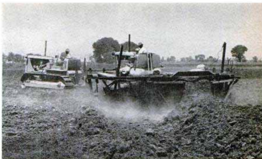
This checking machine scoops up dirt to form a levee along a contour line. It operates like a 16-foot snowplow in reverse
