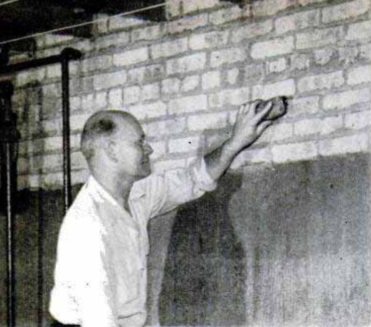
Unpainted wall is cleaned with scrubbing brush and washed down. Efflorescence should be removed by etching and rinsing. Allow walls to dry before painting
