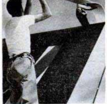
Continuous length of metal goes up over the top of the roof and down the other side
