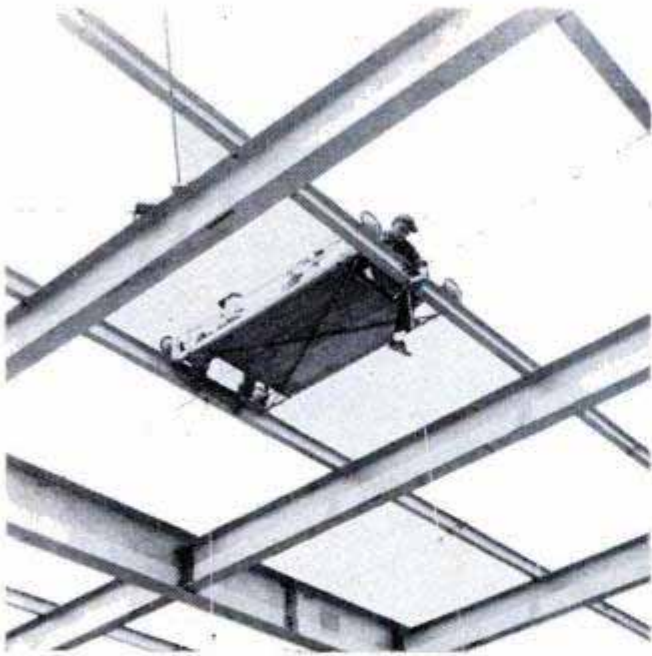
Rolling platform was devised to install fixtures overhead where the plant was without roof or floor
