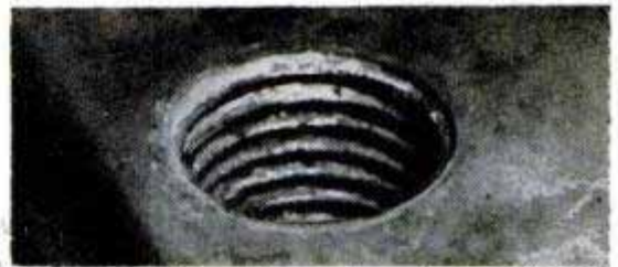
Worn, torn, chewed up, corroded threads that won't hold.
