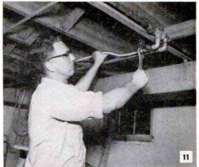
Connecting the copper water line to the cooling unit into an existing water line in the basement
