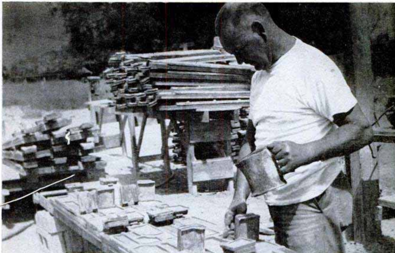
Concrete mixture in various tints, representing Nature's own colors, is poured into sections of rubber mold
