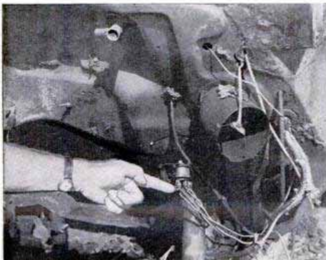
A bared wire in this "harness" caused a fire. New wiring would have been cheaper than repairing damage
