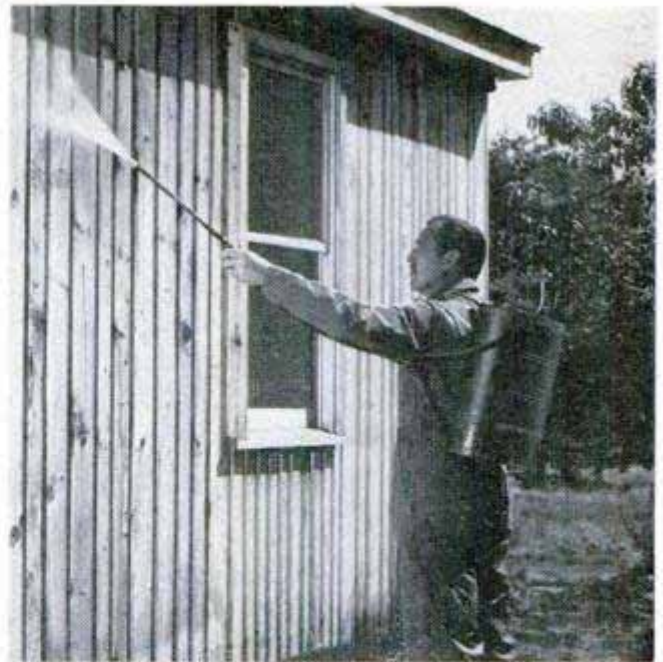
Above, preservative can be applied to an existing structure with portable sprayer. If desired, both stain and preservative may be applied at same time. Mask widows as preservative adheres to glass
