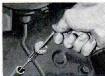
CHECK OIL LEVEL
