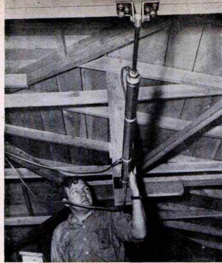
Overhead piston for small doors pulls door open or pushes it shut depending upon direction of water flow
