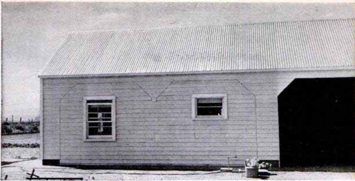
Filled-in doors indicate the owner plans future use of the living quarters as a double garage. Drop siding is a popular material and most of the Deschutes project's roofs are of corrugated aluminum
