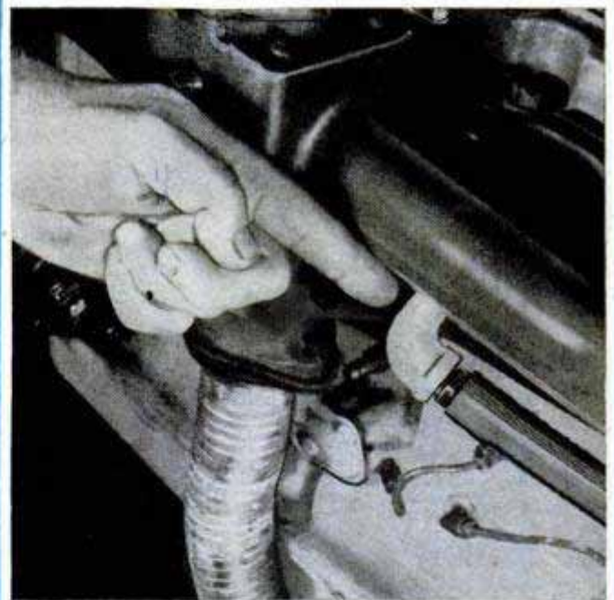
Manifold air bleed is best installed by removing manifold and turning 1/2-in. pipe elbow into tapped hole on underside. Length of 1/2-in. hose leads from elbow to valve under the instrument panel
