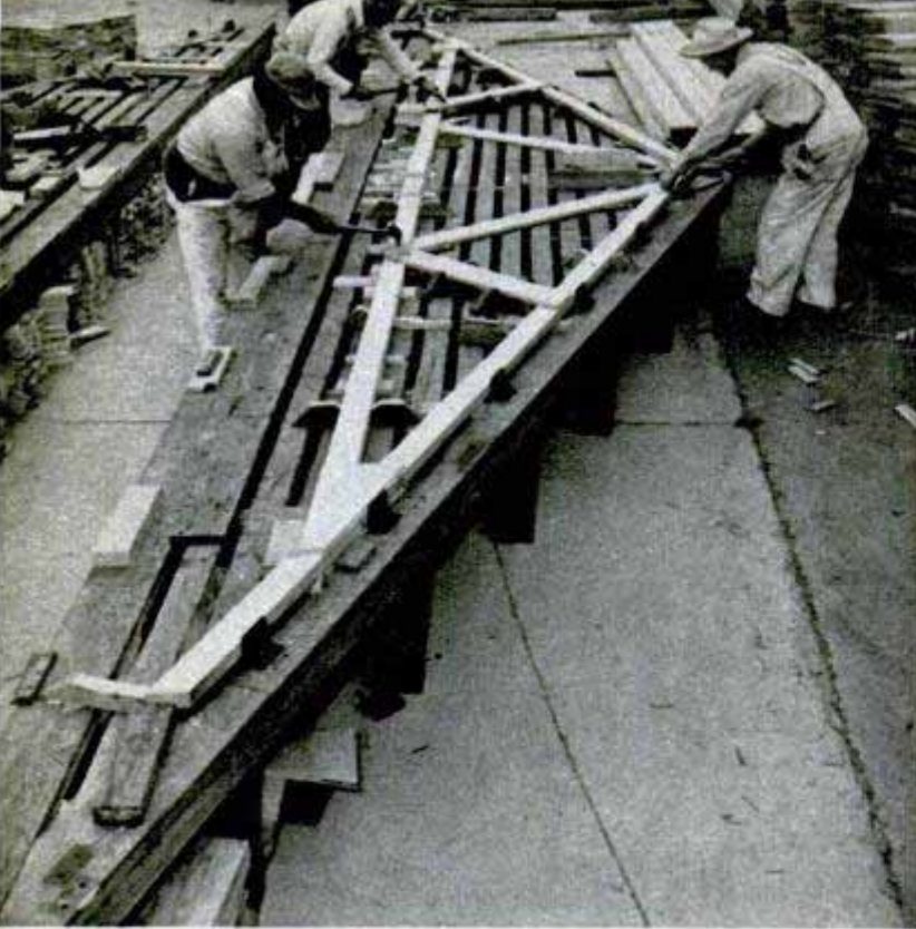
In Nelson's house factory, standard sections of a home are prefabricated. Above, carpenters are nailing a roof girder laid out on sturdy pattern table
