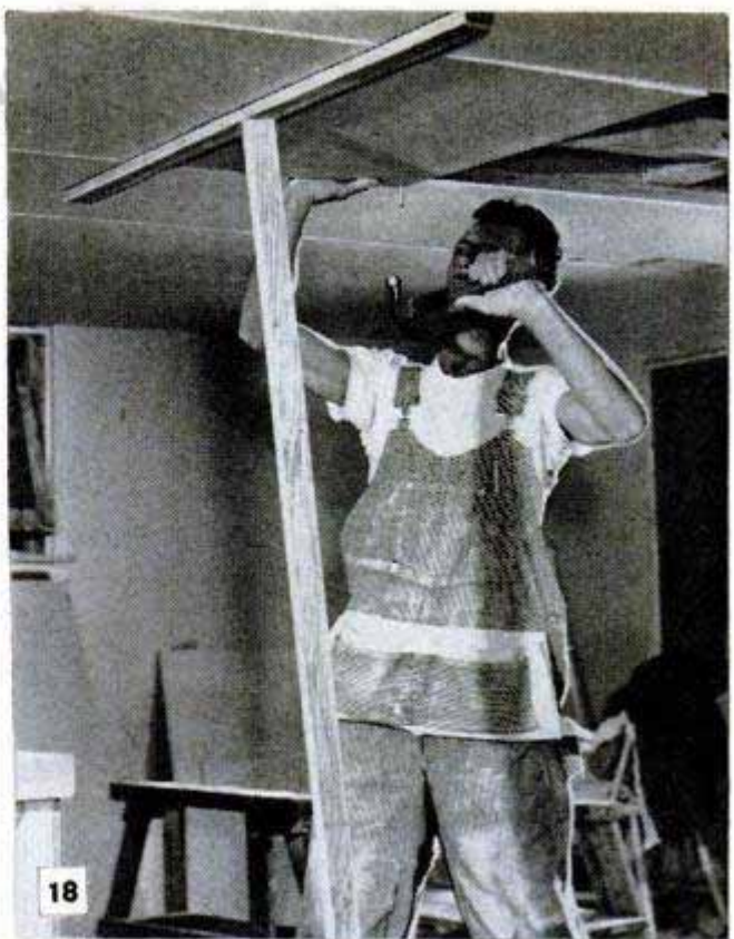
Installing large sheets on ceiling singlehandedly is done by supporting them with a T-shaped brace
