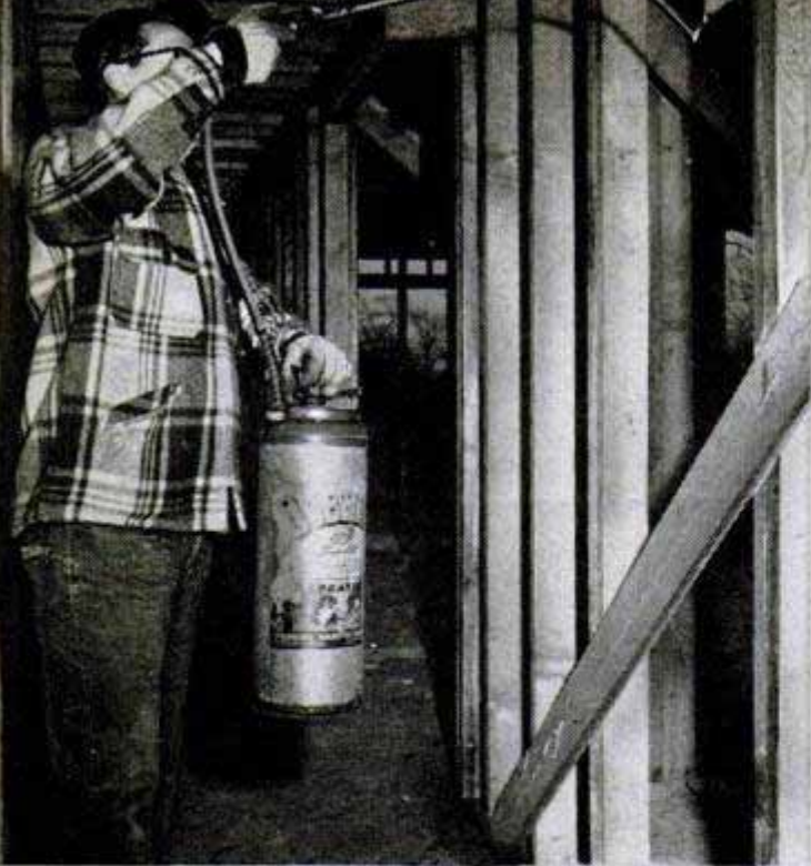
Sether sprays studs of fire wall with water-repellent chemical to protect the wood before painting them with fireproof paint which is water absorbent
