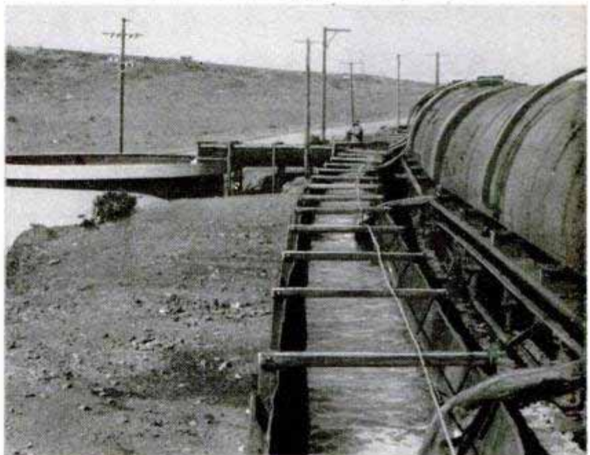
Water trains discharged into gravity tanks at Mount Gipps. From here the water flowed by gravity to Stephens Creek reservoir, 14 miles away. After leaving the reservoir, it filled the city water-supply mains
