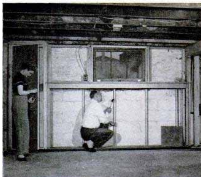
Continuing with the teamwork, Olwen fits a door latch while I install small wall studs in the shelf area
