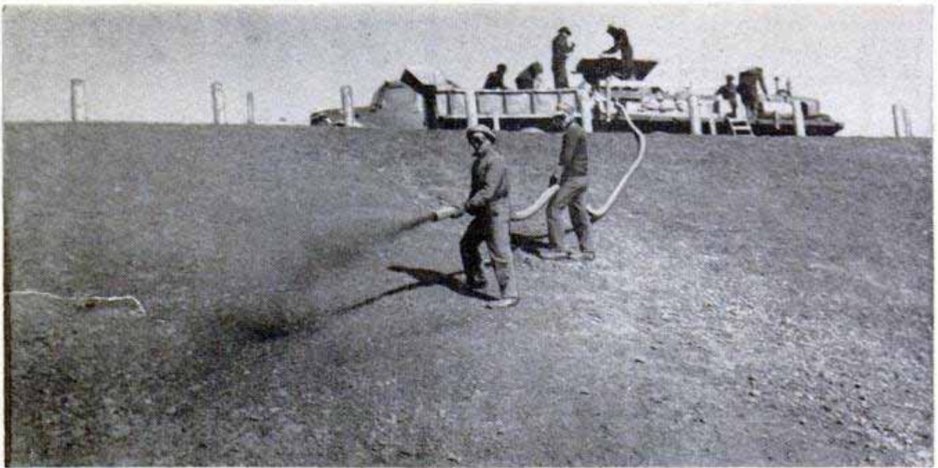
Guiding the flexible blower tube, workmen distribute grassing mixture across a sharply inclined slope
