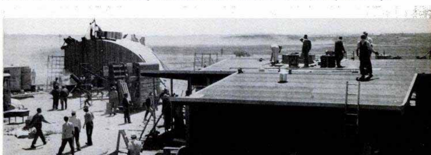
More than 300 workers swarmed over sagebrush land to build the home, other buildings and plant the crops
