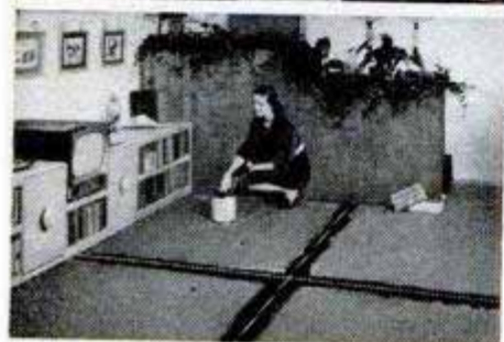
STEP 1... Mrs. Lansing follows the simple instructions. Here she's beginning to spread adhesive over half the play room.
