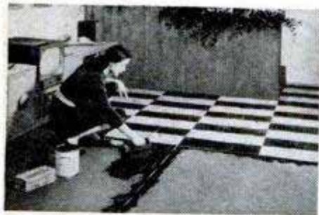
STEP 2... She puts tiles down in place, one at a time. When half the floor is covered, the adhesive is spread over the remaining half.
