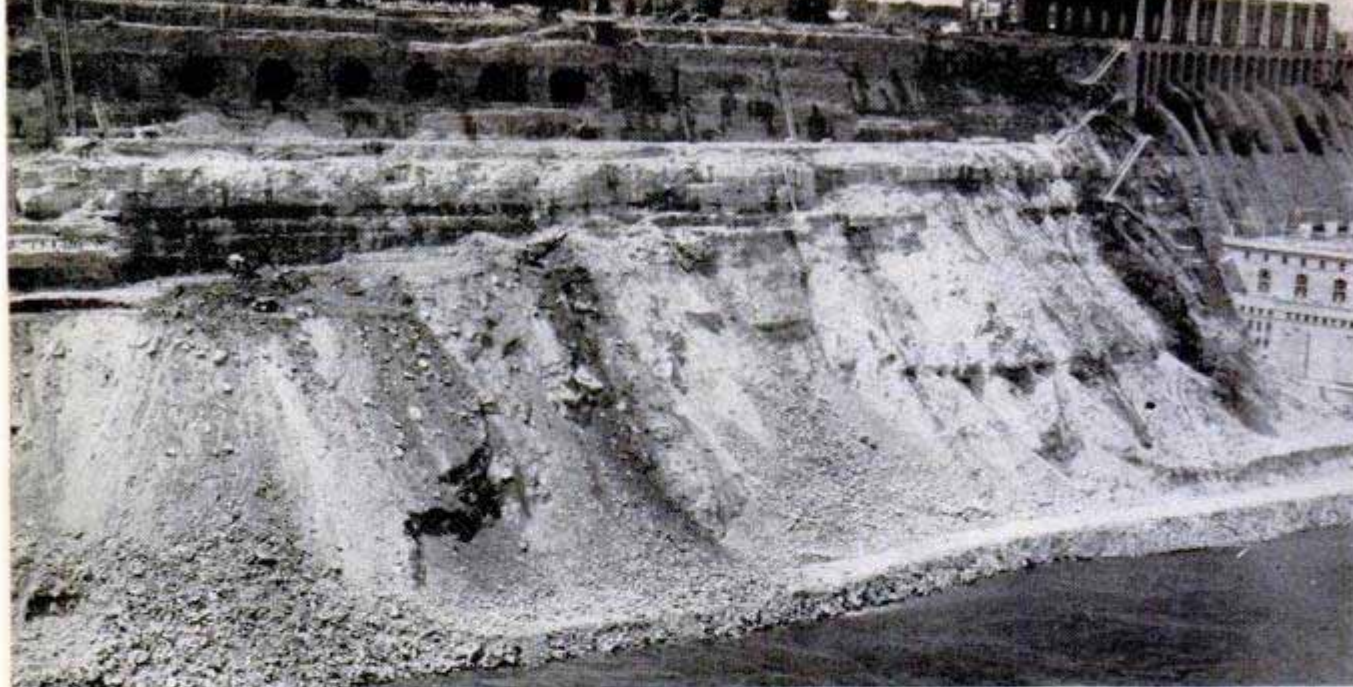
Seven holes near top of cliff will be penstock intakes of new power plant. Existing plant is seen at right
