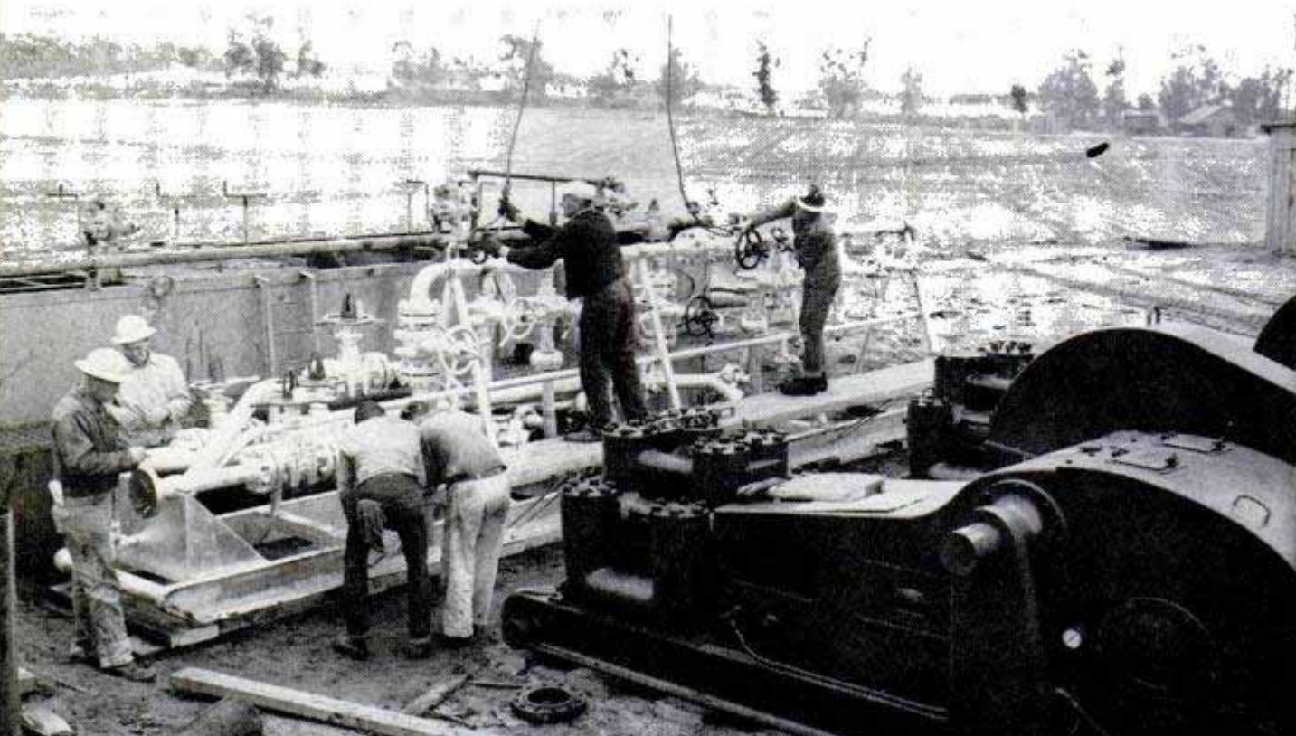
Workmen make connections on the drill's two mud pumps, right. Each unit is mounted on skids for mobility
