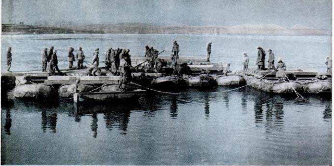
Final link of pontoon bridge is floated into place on the Tong Dong River by the 11th Engineer Battalion
