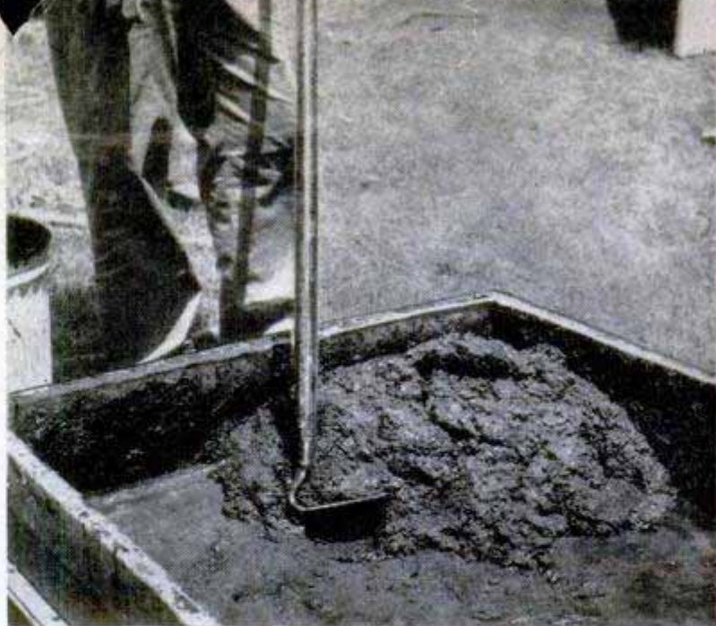
Clay, sand, water and liquid Plasmofalt are mixed into adobe. Mixture then is troweled into brick forms
