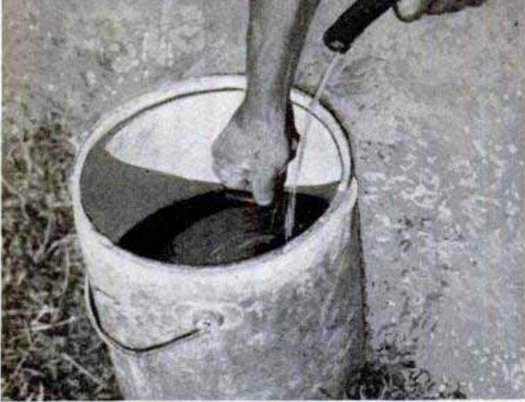
In making \frac{1}{2} -bag batch of 1 : 2\frac{1}{4} : 3 mix, measure 2\frac{1}{2} gal. of water into pail and mark level on inside. Then pail can be refilled with garden hose, as above, for adding just the right amount of water to the mix
