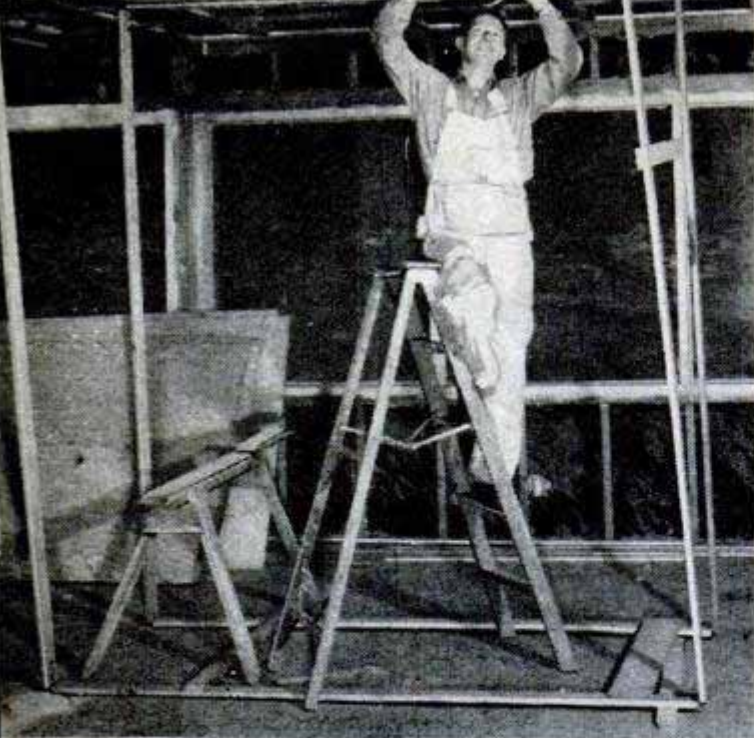
Norman Chapman, my helper, found that a ceiling horse to support the plywood let him concentrate on nailing. Detail at the right shows how to make one
