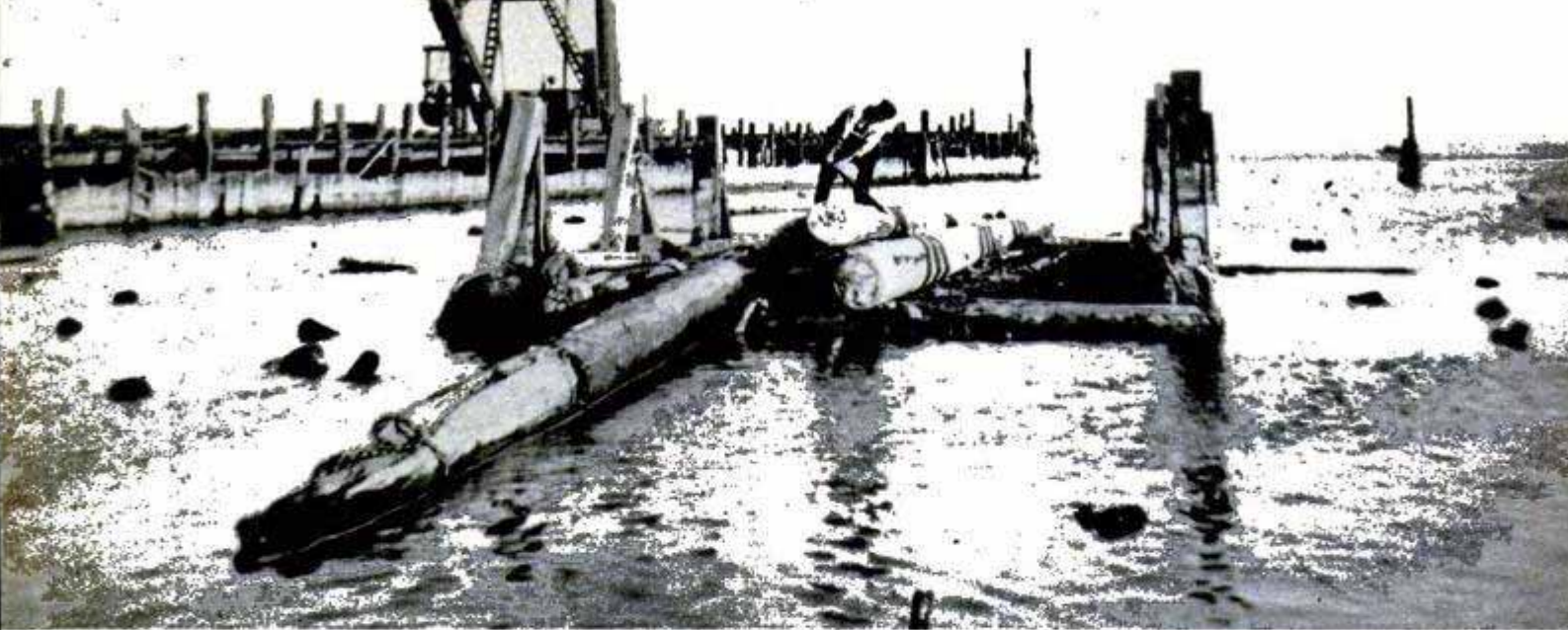
Salvaged piling is dragged off the ungainly "catamaran" by a winch and hauled up on the beach at the sawmill
