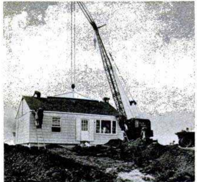
Workmen seal up the joints of the completed house. It was assembled on the site in less than two hours
