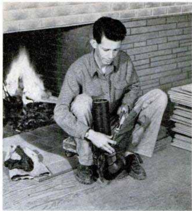
While plumbing can be installed before the subfloor is down, I did it afterwards. Layout plan on opposite page accommodates all future appliances you might consider owning and costs little extra to include now
