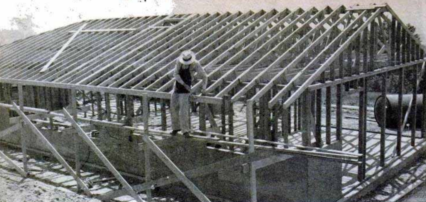
Here I'm beginning to box-in the roof overhang with 2 x 4s which later are faced with clear-grade 1 x 6 boards
