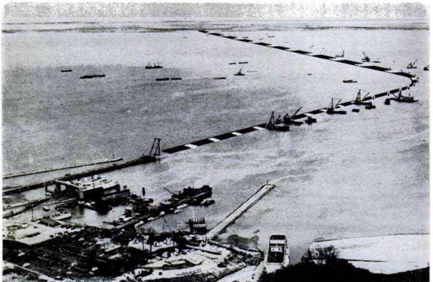
Work along 4.3-mile length of the bridge was not delayed by one lost barge. Sandy Point, Md., is in distance
