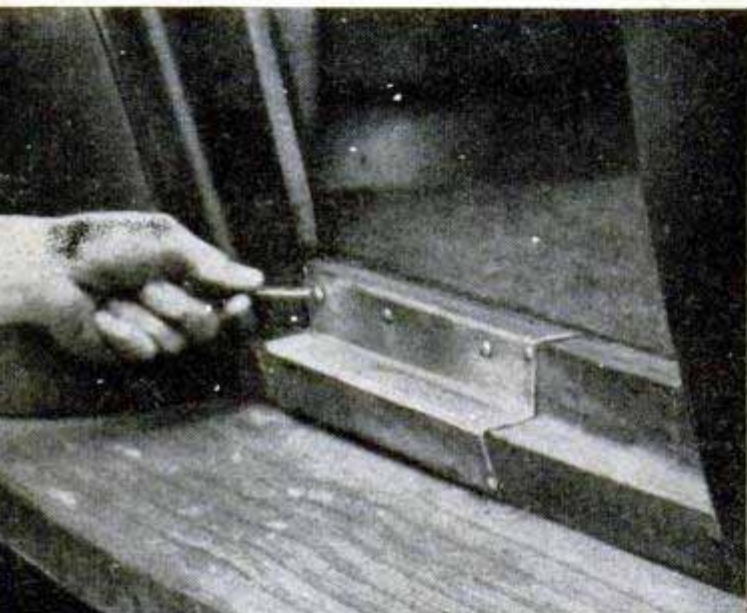
Door-sill patch, which has been bent to shape, is fastened to the car body with self-tapping screws
