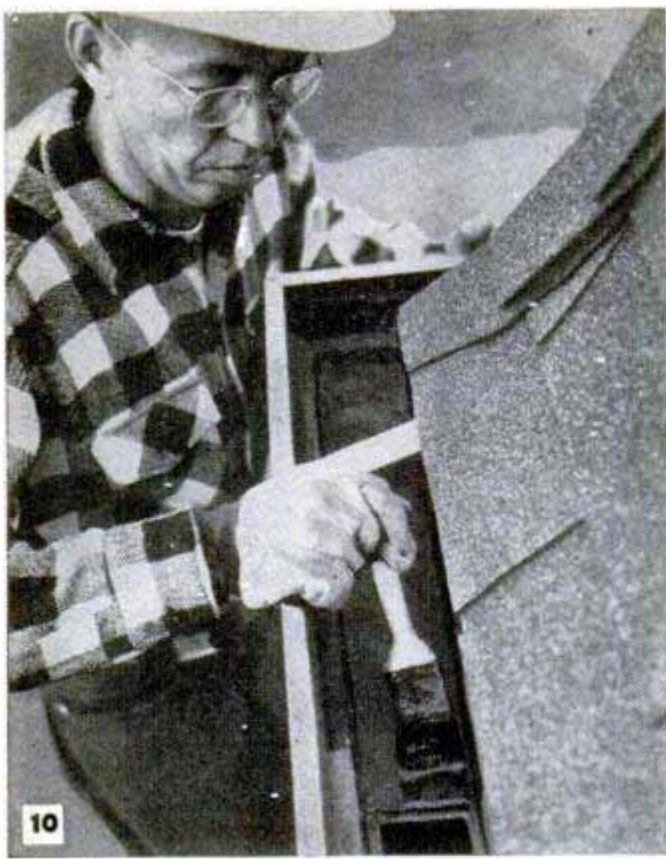
Sheet-metal gutters of all types should be protected with asphalt-base corrosion preventives. After gutters are thoroughly cleaned, material is applied with brush
