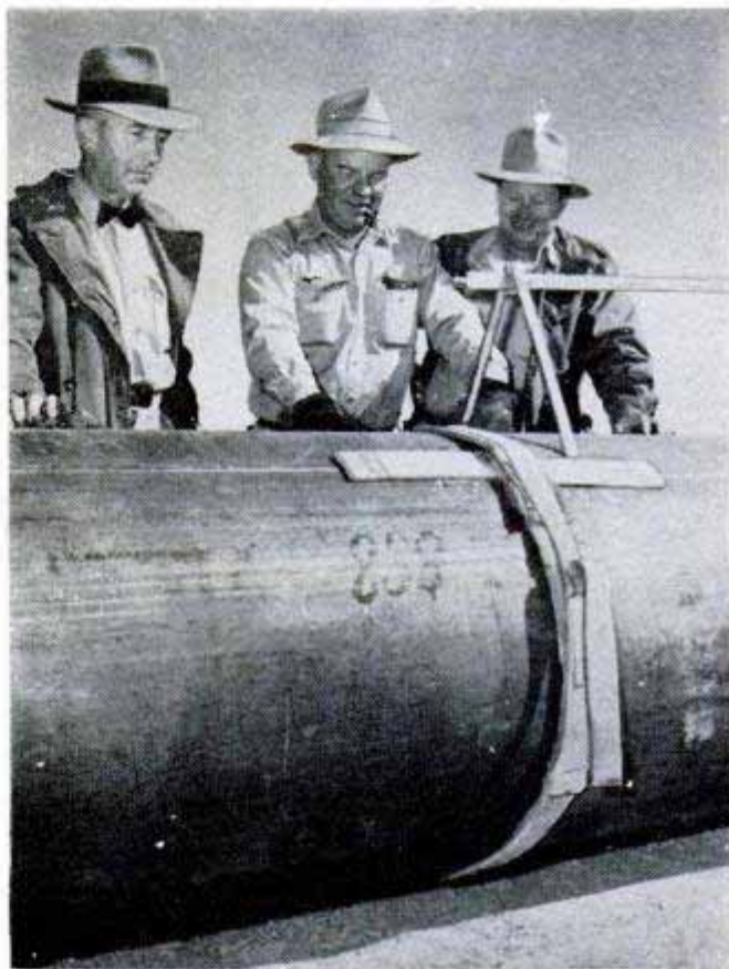
X-ray film is wrapped around weld. Radium salt inside pipe will expose film through any weak spot
