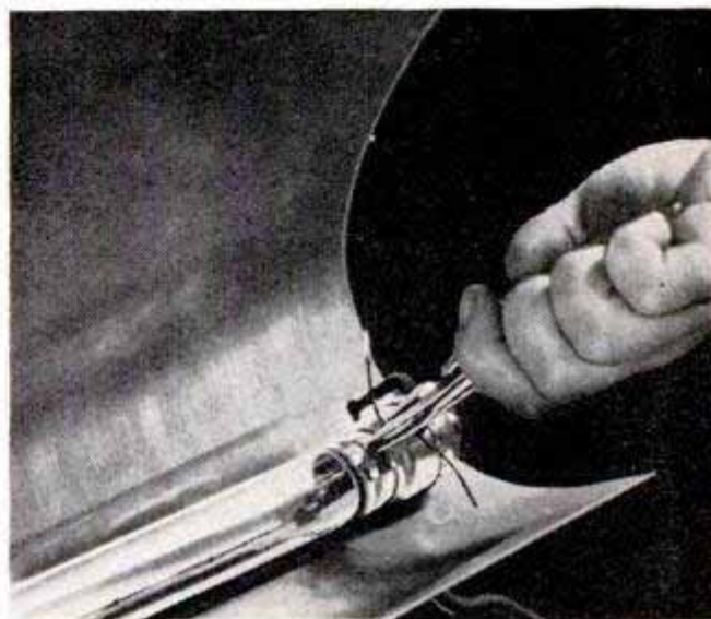
Although socket can be wired in place, it is better to support it in an angle bracket and fixture bushing
