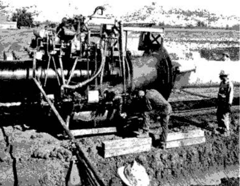
Ingenious machine coats the pipe line with asphalt, felt and paper before it is lowered into the ditch
