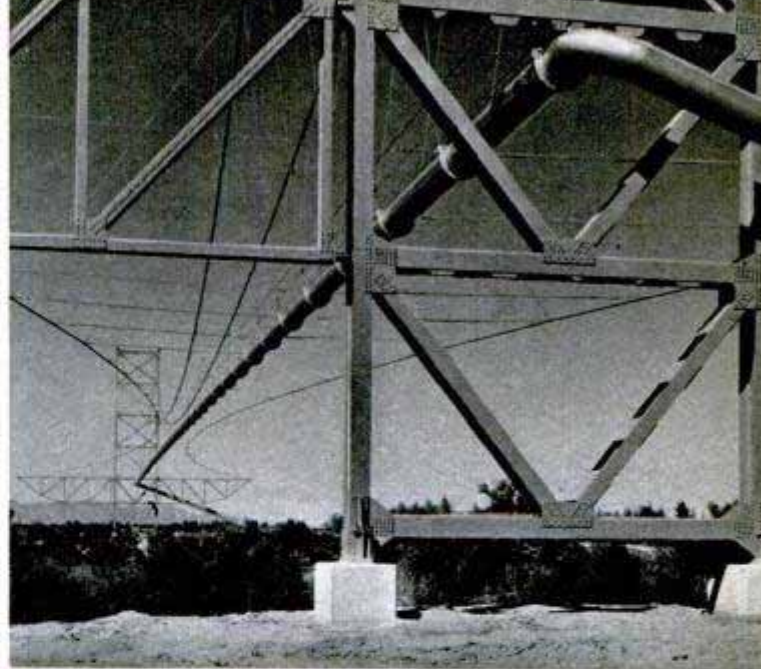
Spiderweb of cables 1200 feet long carries the new West Coast gas pipe line across the Colorado River
