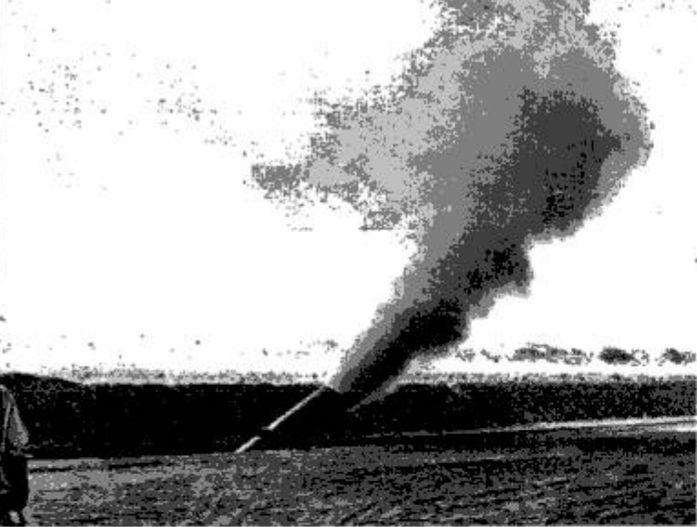
New pipe line is purged of dust and other foreign matter by blowing gas through it under high pressure
