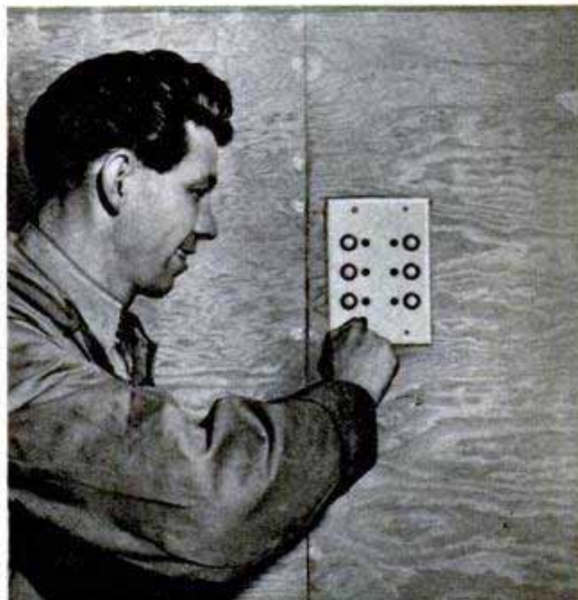
All lights in the house can be controlled by a 24-volt master switch in the bedroom
