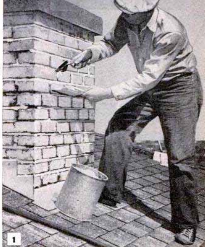
Chimneys frequently need tuck pointing as their location subjects them to all damaging weather elements
