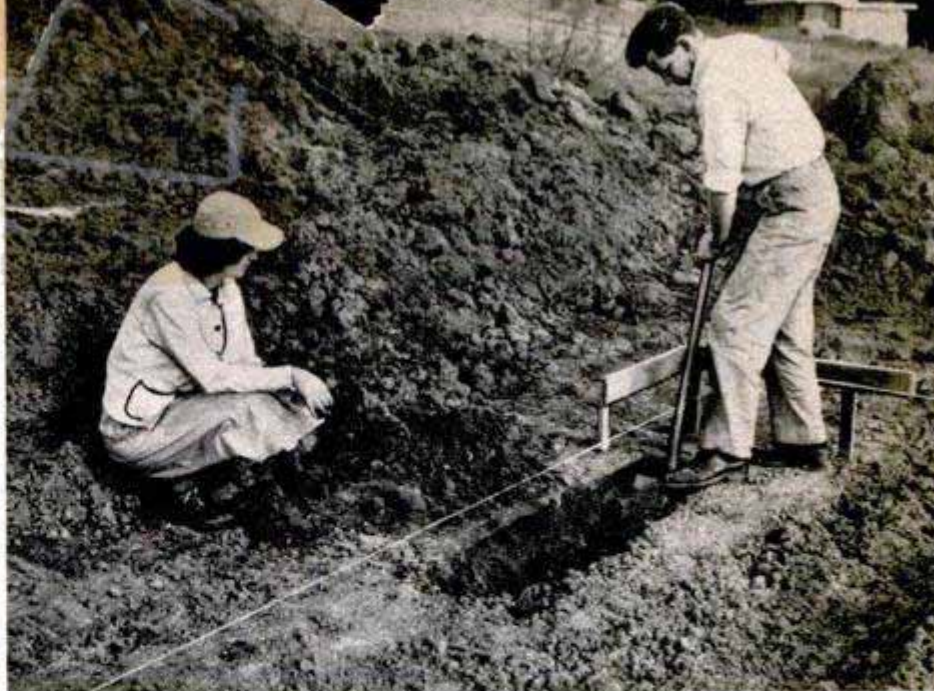
After a few turns with the shovel, Tom advises: "Don't be afraid of hiring power machinery for the excavation." Mrs. Riley kibitzes
