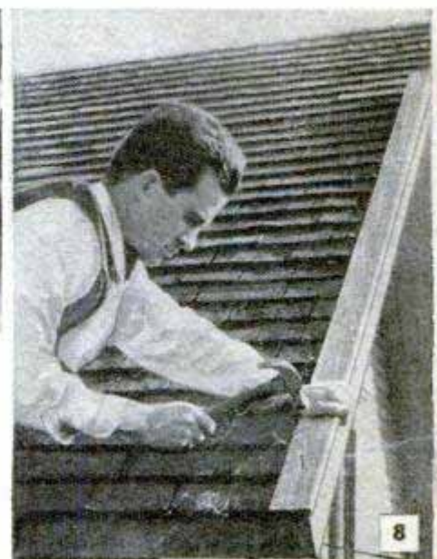
8 DRIP EDGE OF 26-GAUGE SHEET METAL GIVES PROTECTION AT EAVES AND RAKE
