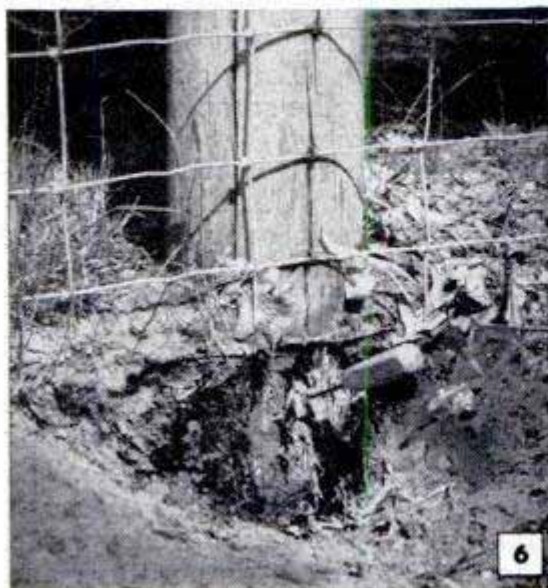
Decay of some untreated posts progresses to this stage in three to five years' time
