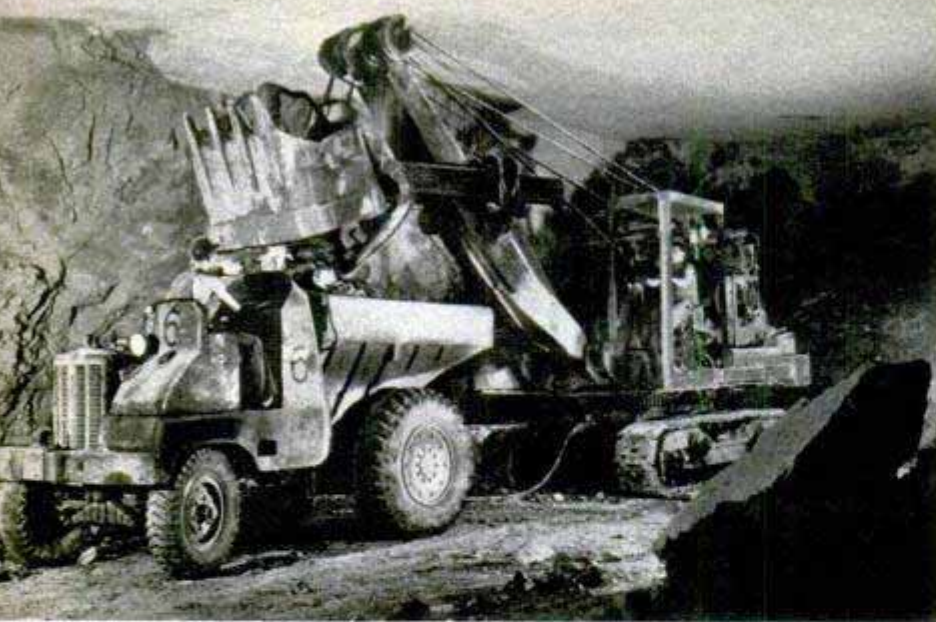
All the huge electric shovels used to load the limestone had to be carried below in pieces, then reassembled by mechanics
