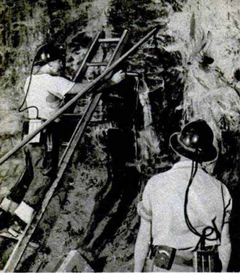
Placing dynamite in hole drilled in rock face. It is set off remotely after last man leaves the mine
