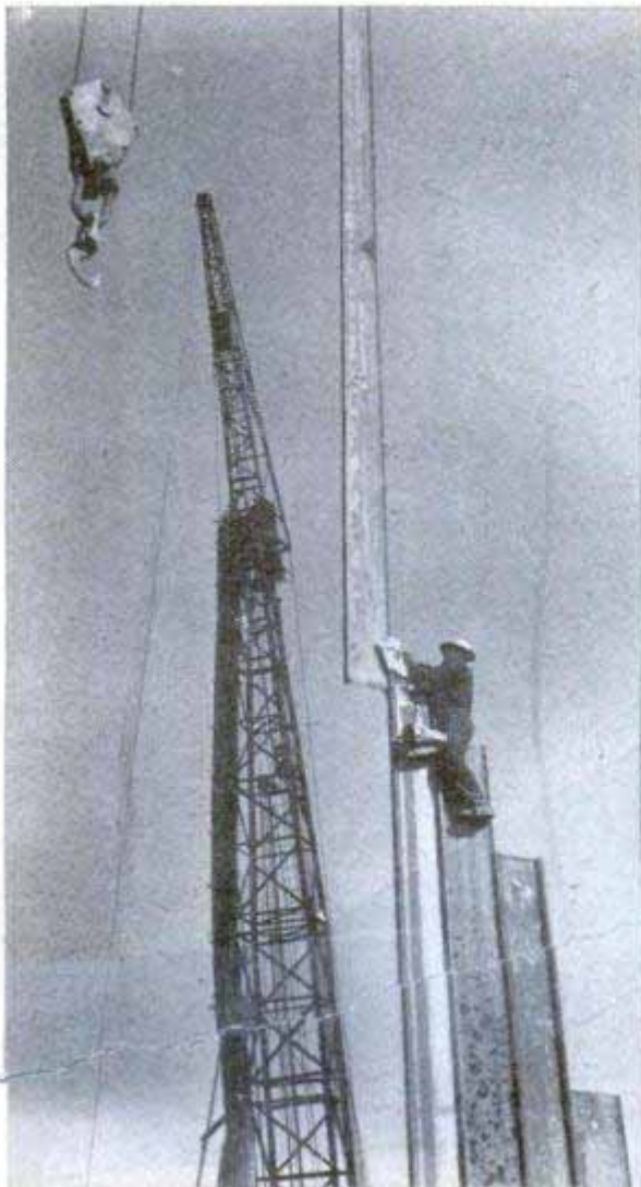
Above, lowering one of the 79-foot piles into position prior to driving. The piles interlock
