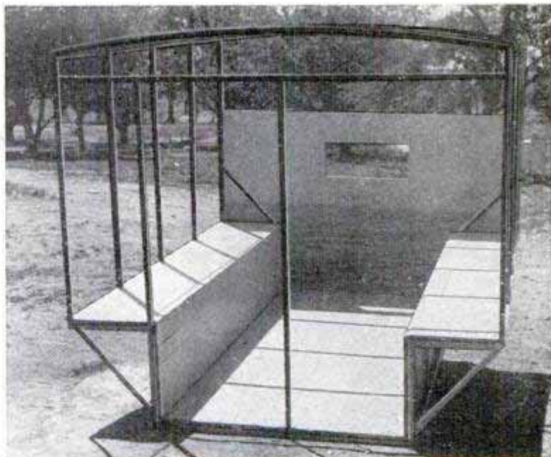
The angle-iron frame of the "pickaback" trailer body with the floor and front panel installed. Note the front window opening
