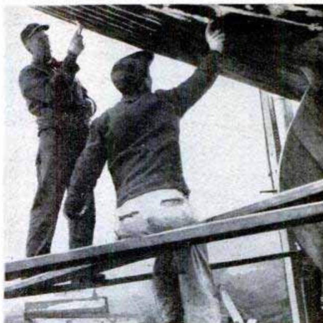
Seam cement is forced into calked seams to make a smooth watertight job before sanding and painting
