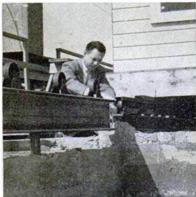
Finished home, still on rollers, moves over a pit so the house-moving equipment can be installed
