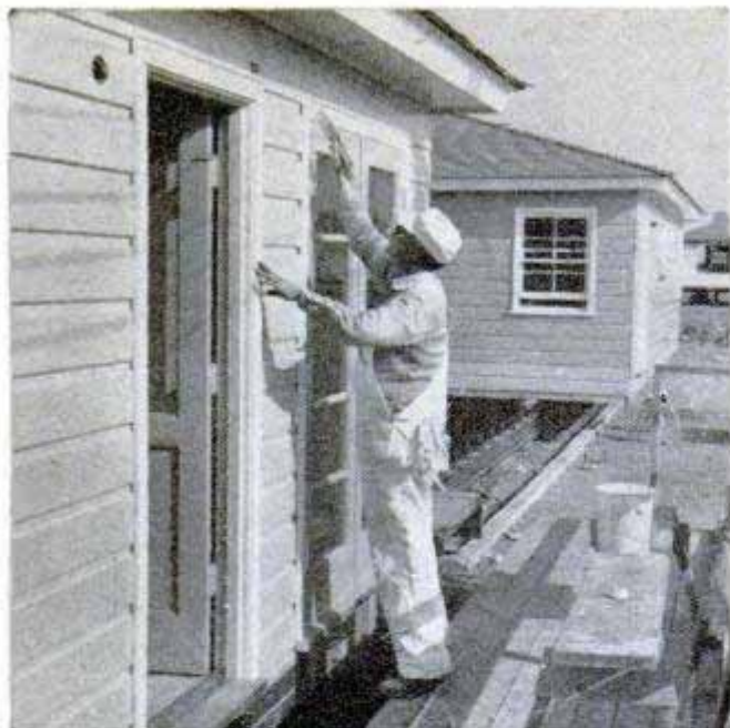
Near the end of the line the house receives three coats of paint. The purchaser chooses the colors
