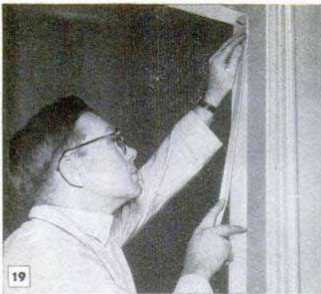
Masking tape is used to get straight meeting line on swinging-door frame where two colors are used
