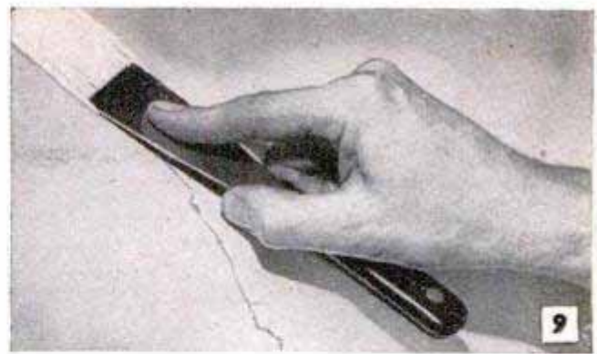
Use a stiff putty knife to press the crack filler into holes, dents and cracks in the plastered walls
