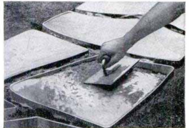
4th. Molds are filled level with concrete, tamped and troweled. Straightedge is used to rake off excess
