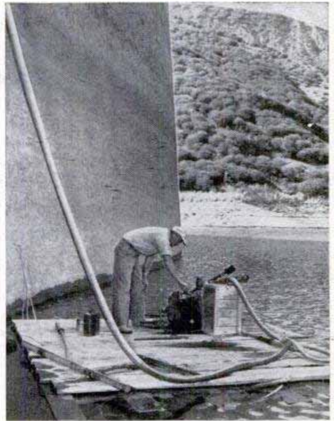
Pumping unit on raft behind Gibraltar Dam supplied water to local residents during California drought
