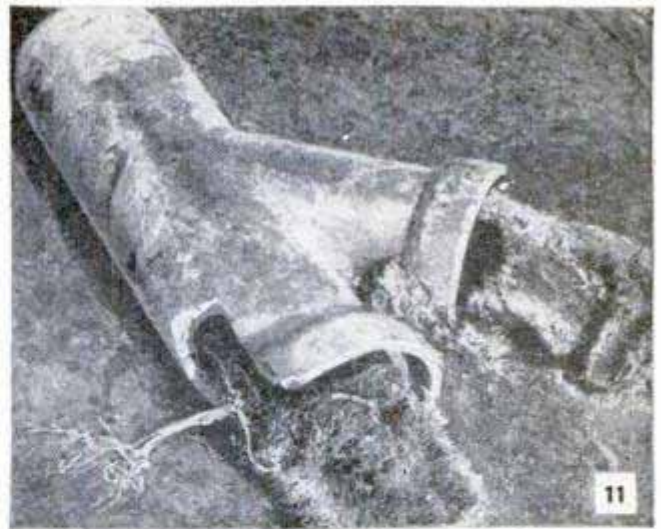
A sewer tile completely clogged and even broken by the dense growth of tree roots, some \frac{1}{4} in. thick
