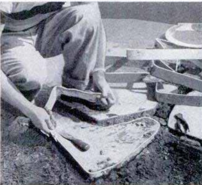
5th. Removal of the sheet-metal molds is easy. Just cut the wire holding the ends and jerk the strip free
