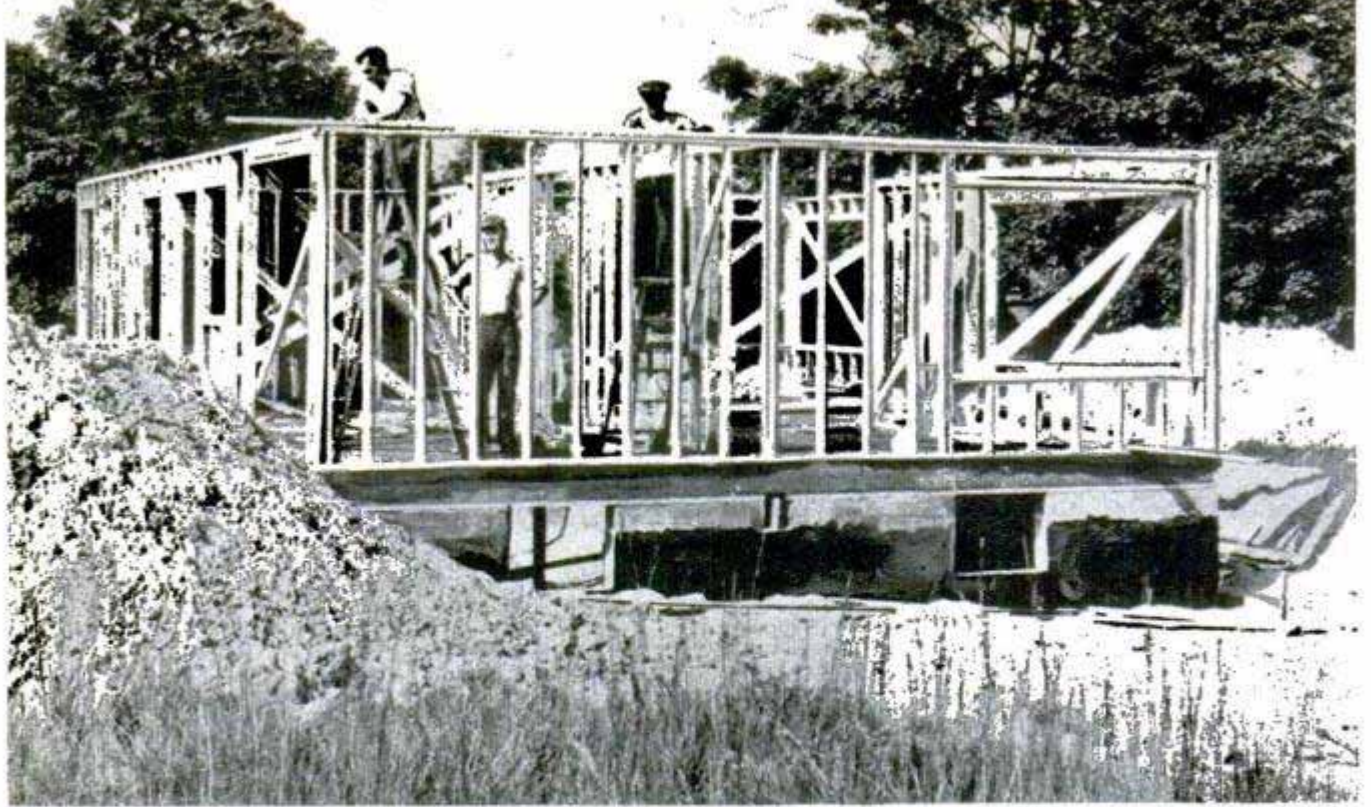
After the third Saturday's work, the Rutherford's house was framed up and ready for the second-floor beams
