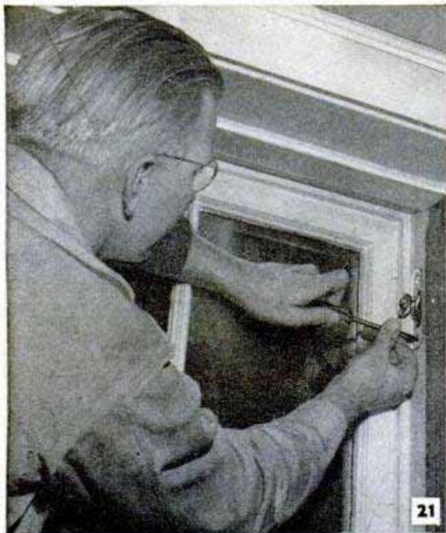
Counterweights may be replaced with spring-type sash balances. These are installed in slots for pulleys, and metal tape is attached to hook on edge of sash
