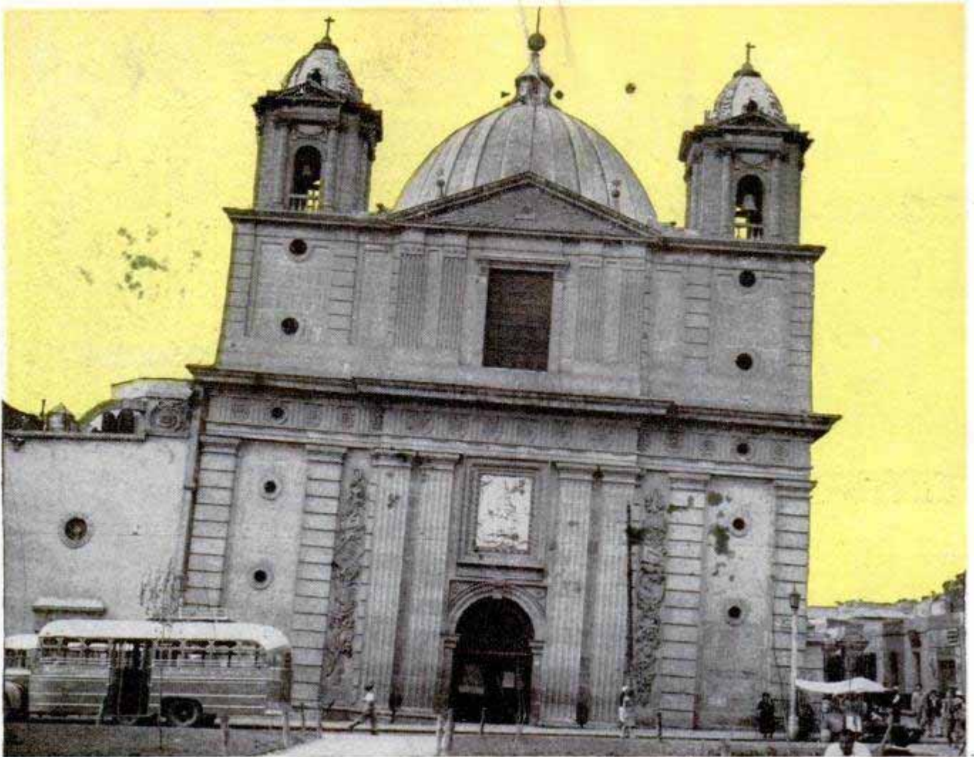
This 300-year-old church has tilted three feet from the vertical due to uneven settlement of the soft soil
