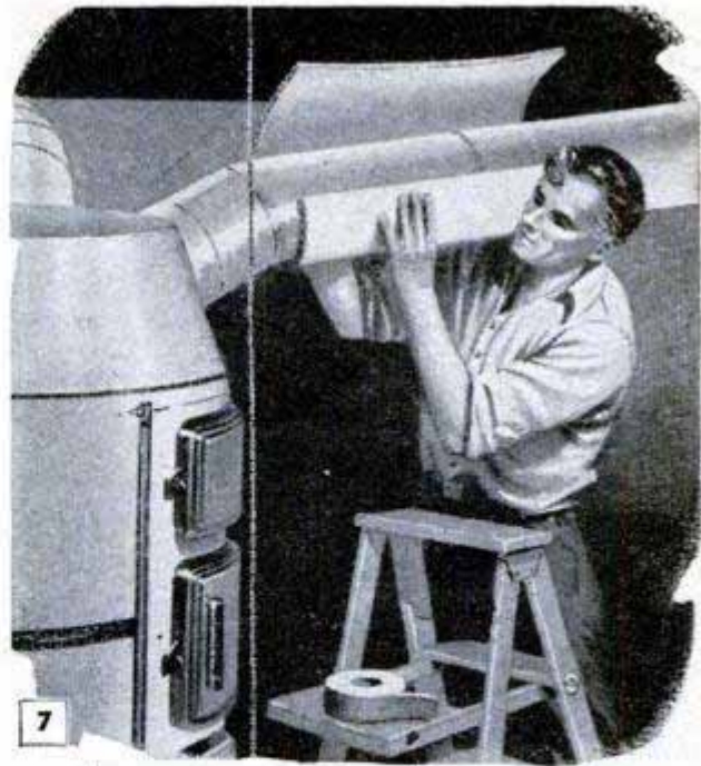
Corrugated insulation on warm-air ducts stops any heat loss to the basement. Seal joints in the covering with gummed paper or cloth tape applied tightly
