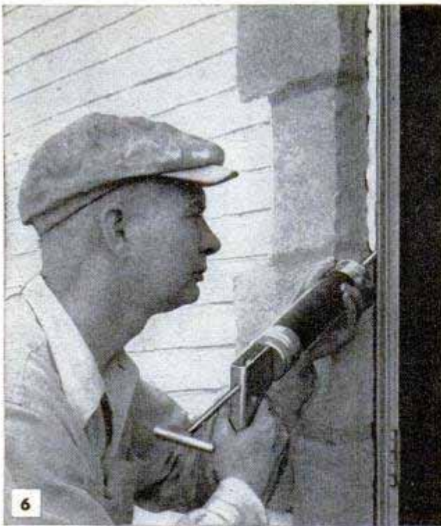
6 Caulking seals open joints where doors and windows join masonry. A gun applies it easily and quickly
