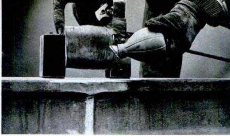
Completed welds are checked by magnetism. Pattern of iron filings on weld under electromagnet reveals any invisible flaws in joint
