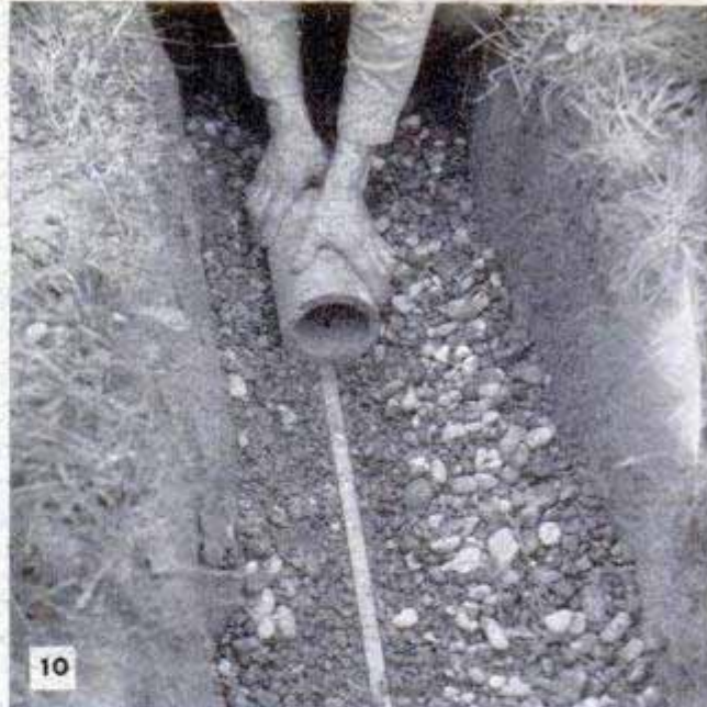
In heavy soils where the natural drainage is slow, disposal tile should be embedded in washed gravel
