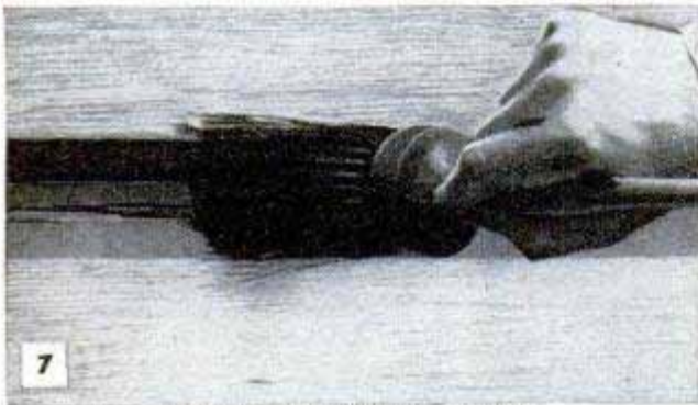
7 FIRST BRUSH DUST FROM CRACKS
