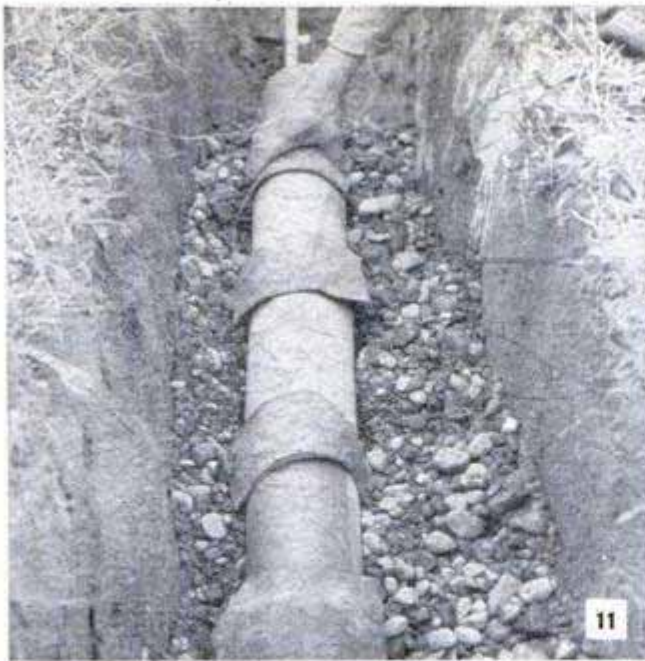
As the open-end tile are laid, each joint is covered with a rectangular piece of extra-heavy tarred paper
