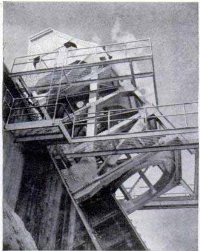
Frame holds motor pointing downward at angle of 60 degrees to avoid damaging a natural-rock sluiceway
