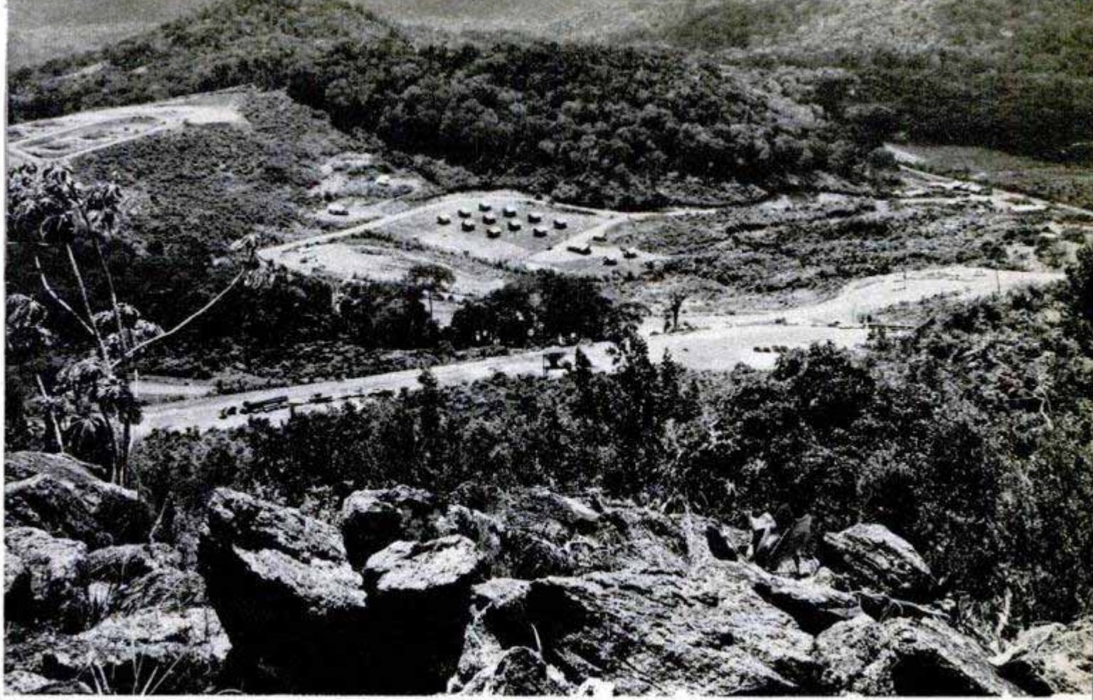
Workers are carving modern road and railroad out of this jungle. That's a labor camp on side of mountain
