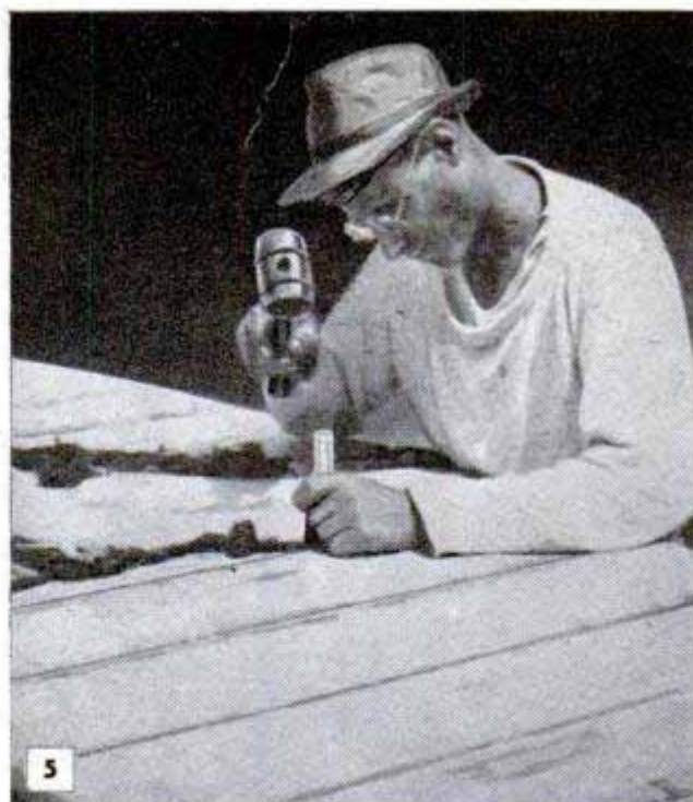
Recalcing periodically will assure a tight, dry boat and add greatly to the life of bottom planking. Important thing is to calk joints uniformly
