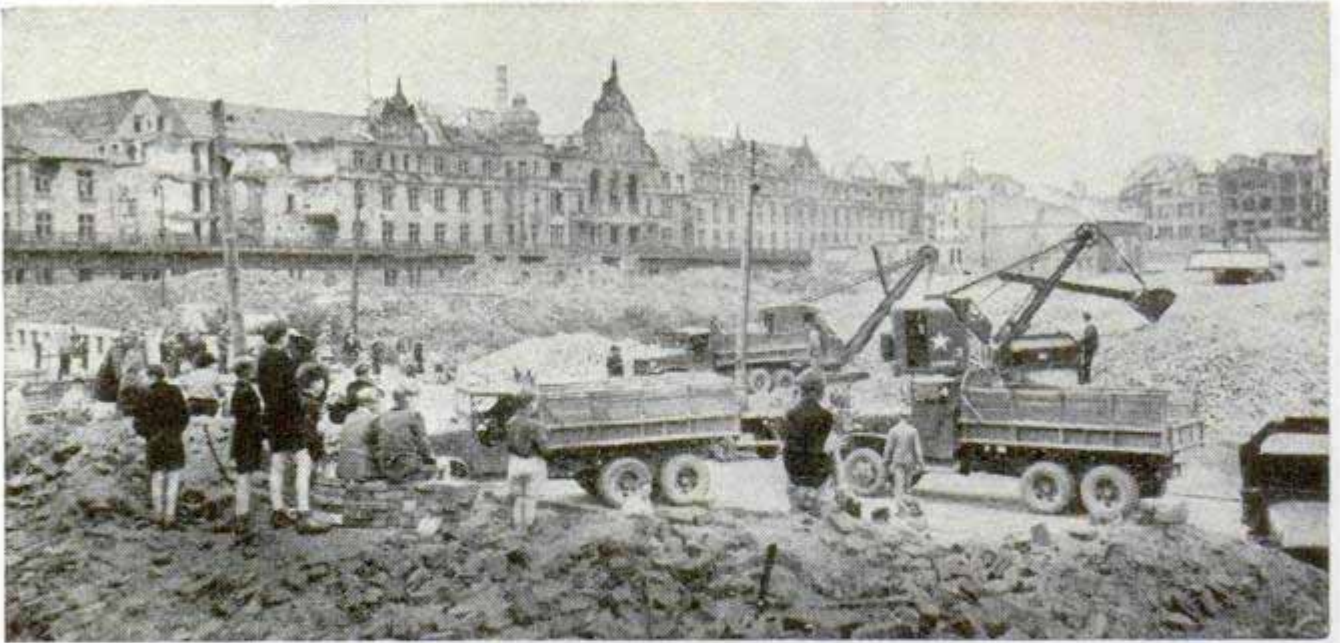
Children seated on brick rubble look on curiously as bulldozers and trucks work on new lift strip at Tegel
