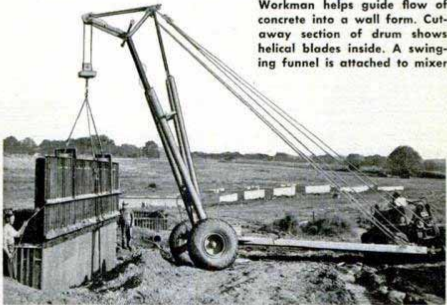
After 24 hours the bolts are removed and a crane lifts the frame from the hardened concrete. Bolt holes are plugged to make wall watertight.
