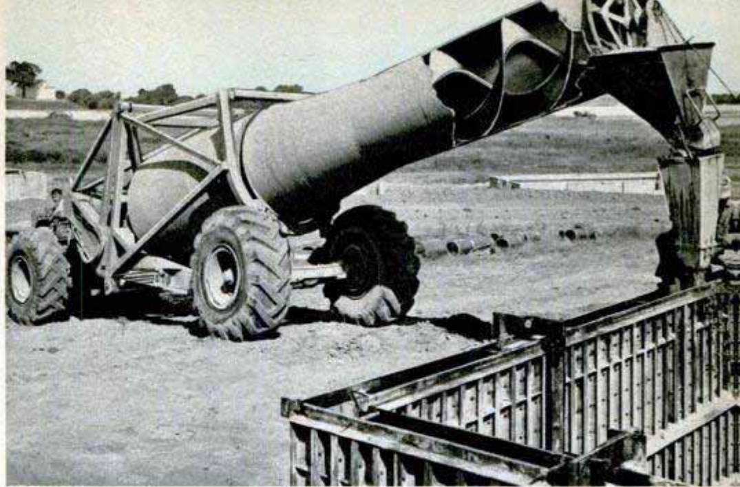
Workman helps guide flow of concrete into a wall form. Cut-away section of drum shows helical blades inside. A swinging funnel is attached to mixer.
