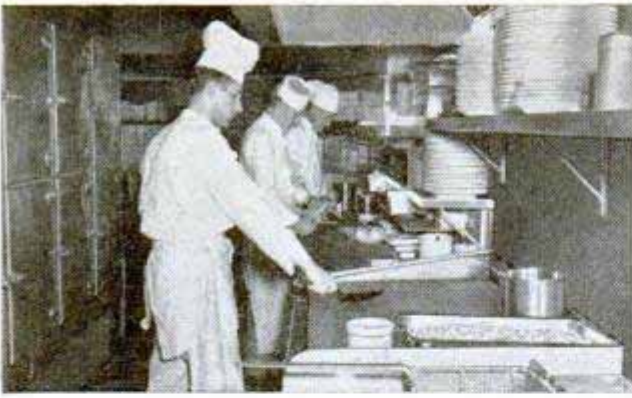
More than 60 orders of fried chicken can be cooked simultaneously in the two identical kitchens. Below, the central cooling plant is a maze of refrigeration units. All the glasses are chilled before using
