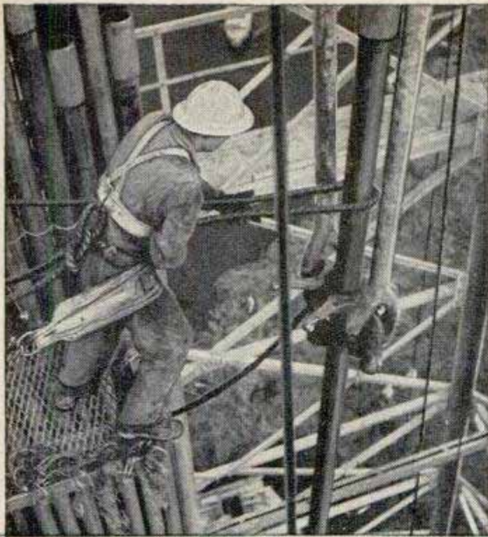
Working 125 feet above the derrick floor, a worker manhandles a 135-foot stand of 5-inch pipe
