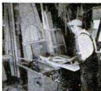
A Delta Unisaw* at the job-site saves time and cuts costs for this builder.
