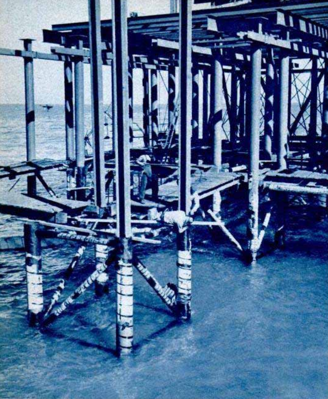
Welders secure the pilings which will support more than an acre of working space. The pilings are driven to an average penetration of 200 feet
