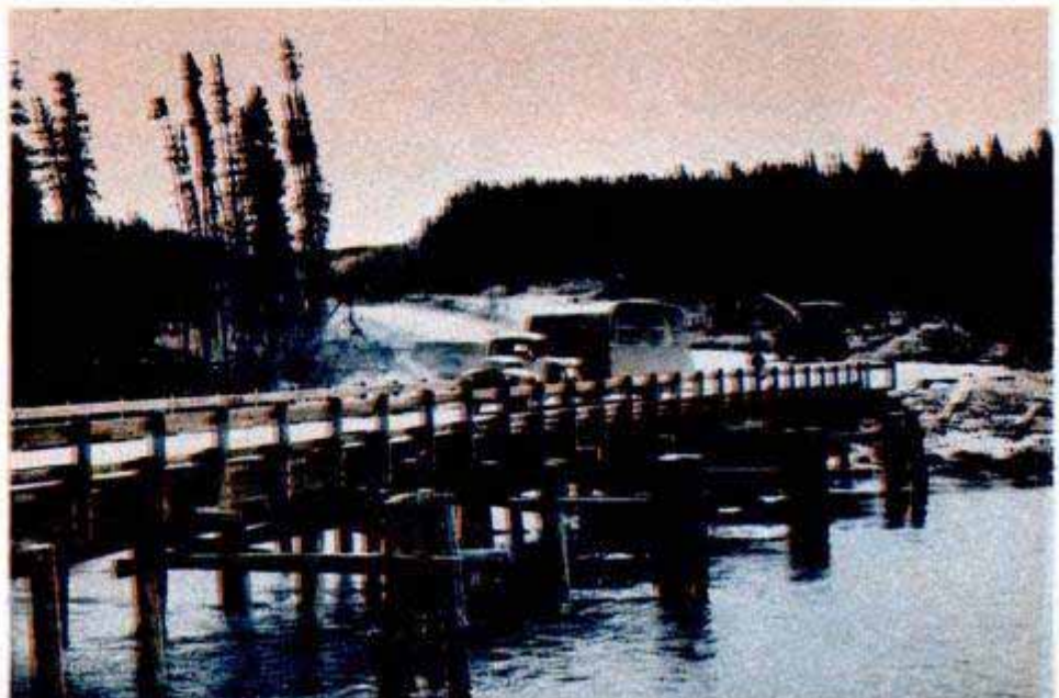
Scene of the worst single washout during 1948, the wooden-pile bridge over the Rancheria River had just been restored when this was taken
