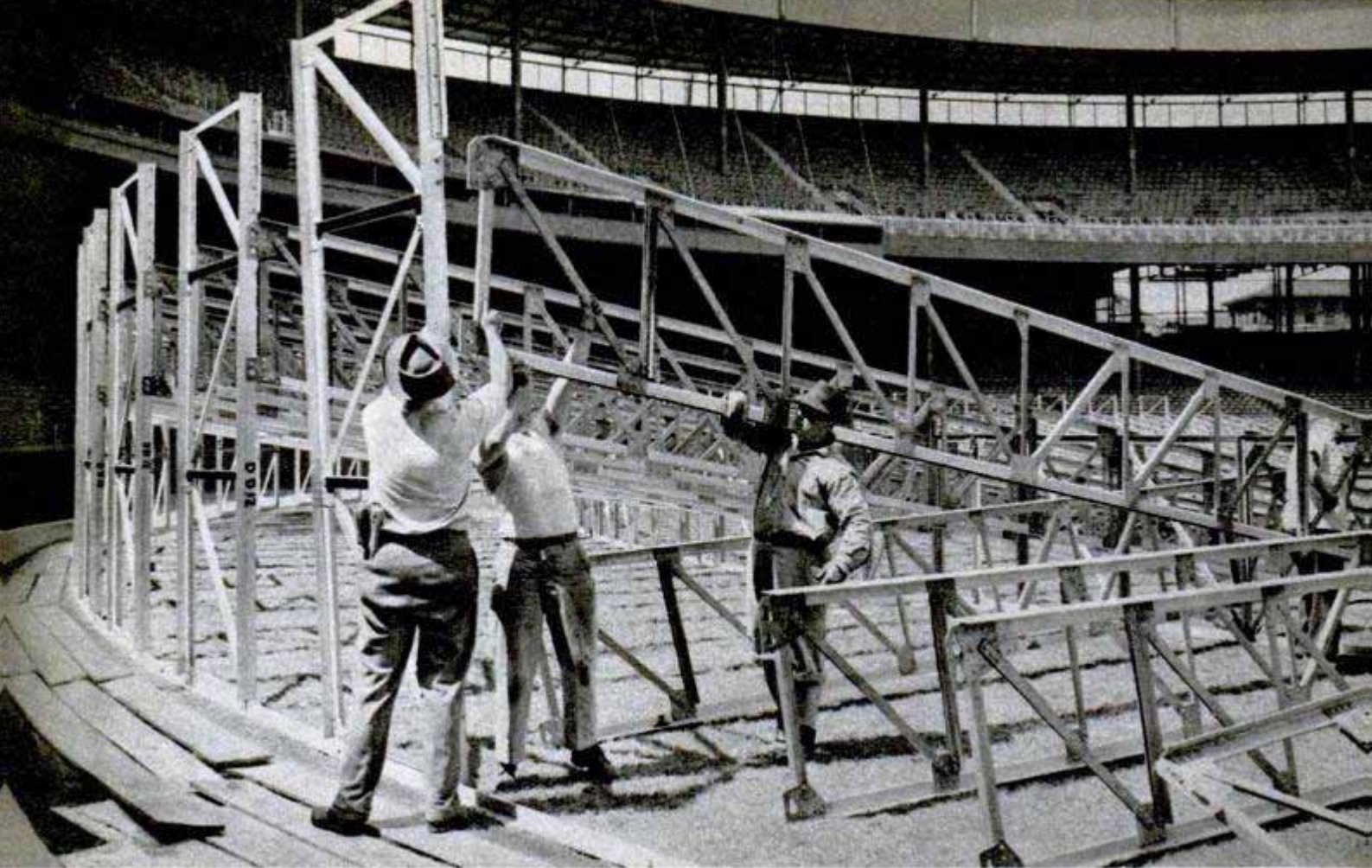
Framework for the oval consists of aluminum trusses secured to vertical members by stainless-steel fittings. Putting together the track is as simple as assembling a child's building set—it just takes more time and labor
