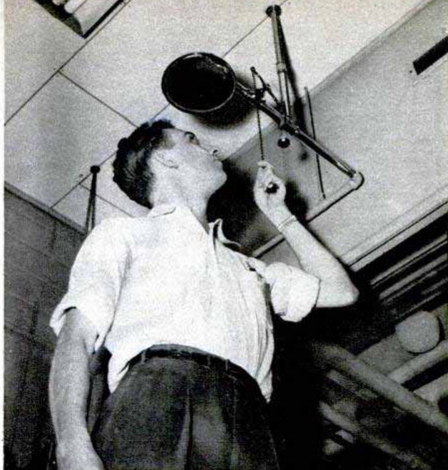
In the petroleum lab is an emergency shower. In case of explosion or fire, worker pulls handle to flood water completely over his body
