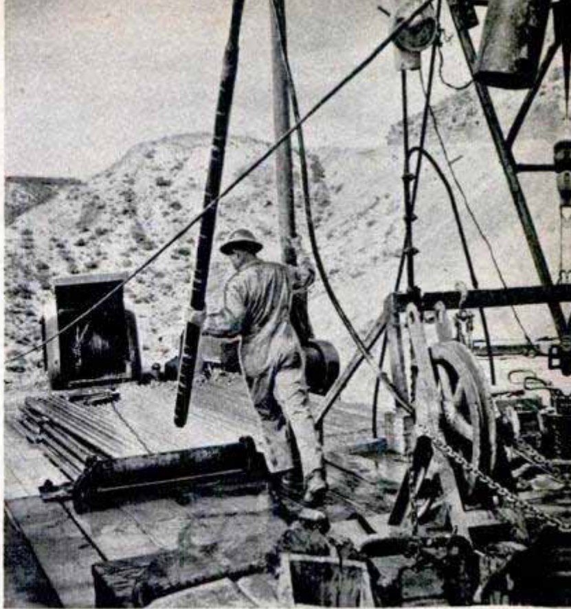
Electrode, being guided by driller, is lowered into the shaft to determine oil potential of the new well
