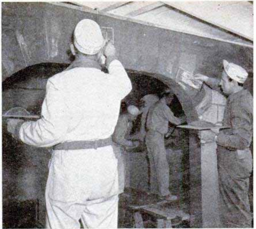
Above, workmen form rough stones from the mixture. Left, air gun sprays stone particles on the surface
