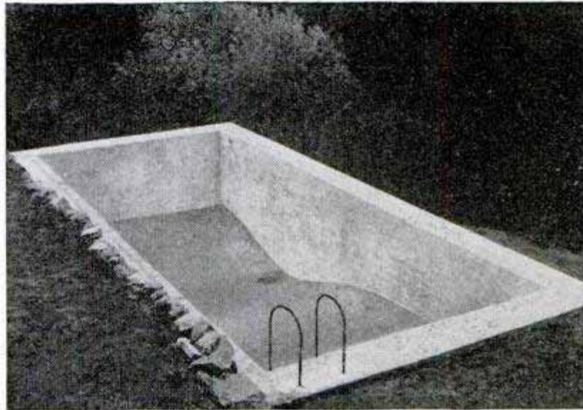
This view shows the pool poured, the forms removed and drain installed. Walls take less concrete when bottom of pool is sloped
